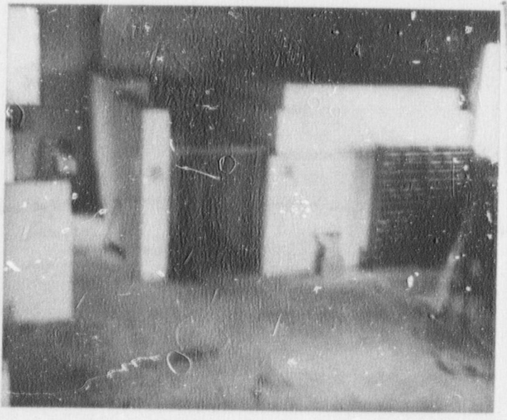
Att. 1 west crack
