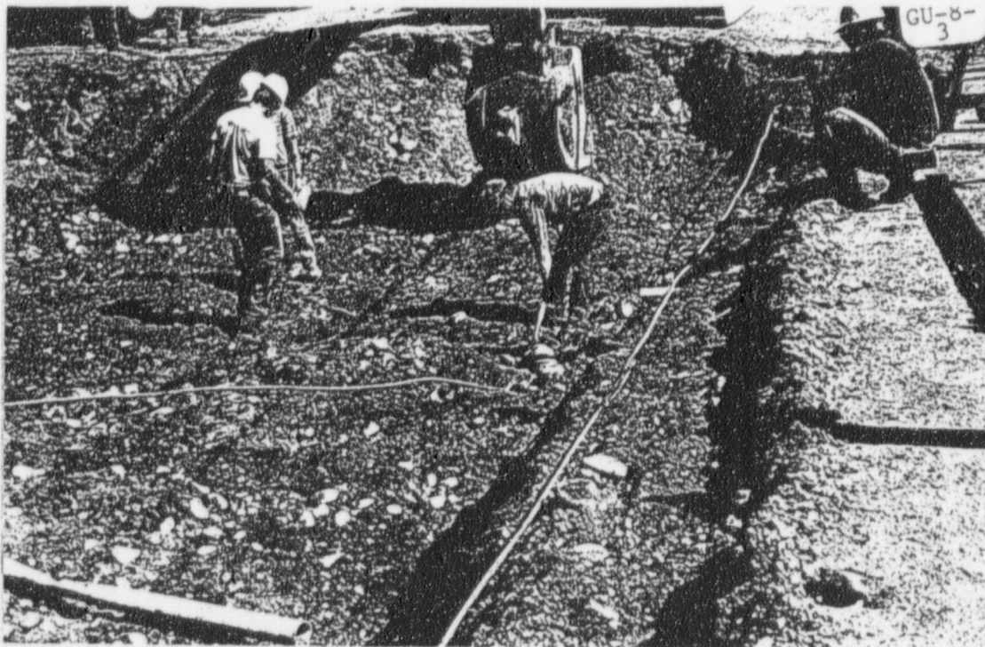
Broken Water Line at STA 3+30.
