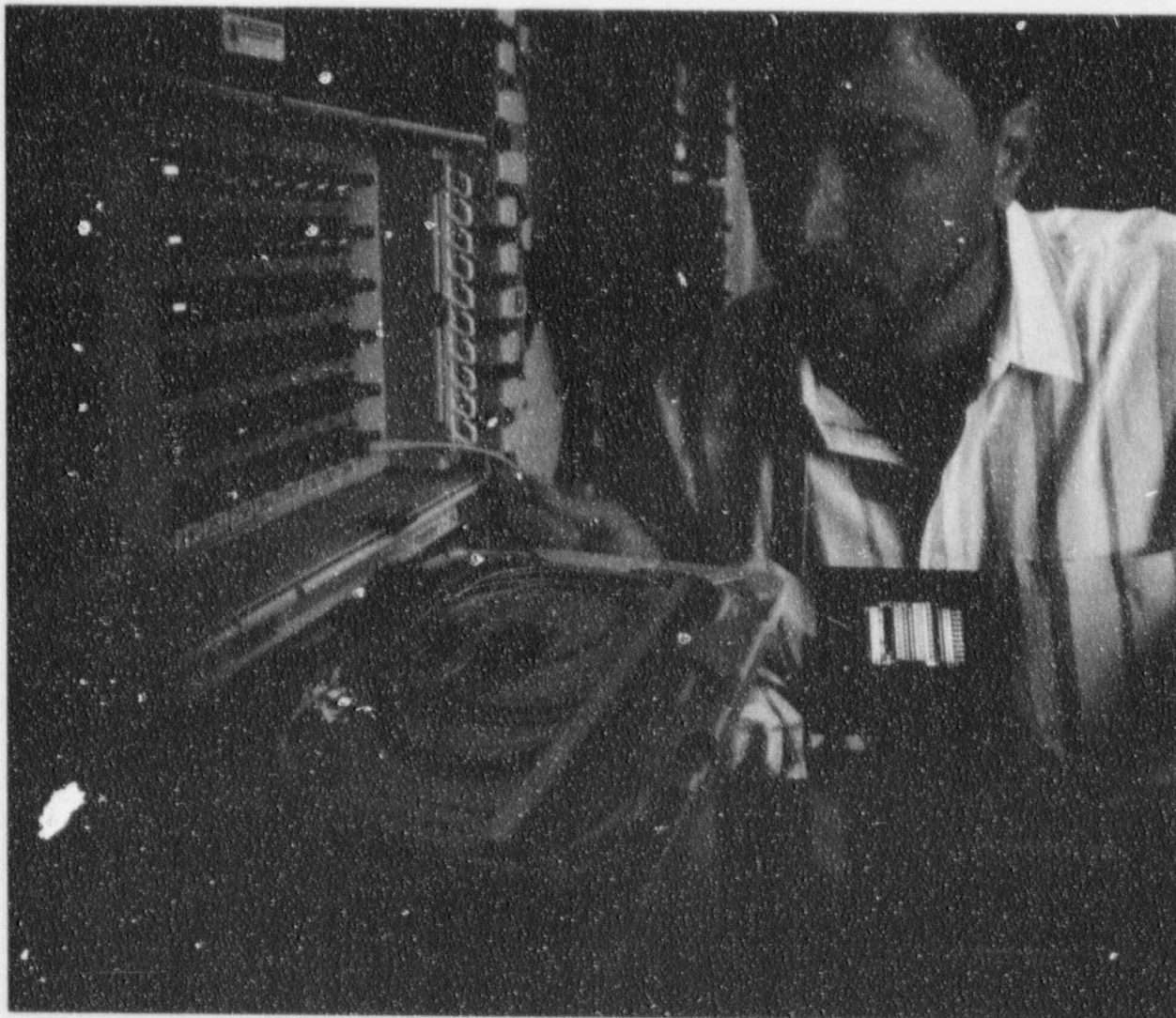
Karl Urbanski, Tester III, inspects fiber optic cable on the distribution rack which serves as a terminal for the glass strands which transfer information between CPS facilities.
