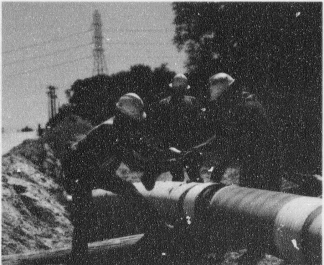
Doyle Haese, Gas and General Construction Inspector, monitors the installation of a 16-inch gas main part of the second outer loop which will encircle San Antonio by the year 2000, making both gas and electric service available in north Bexar County.
