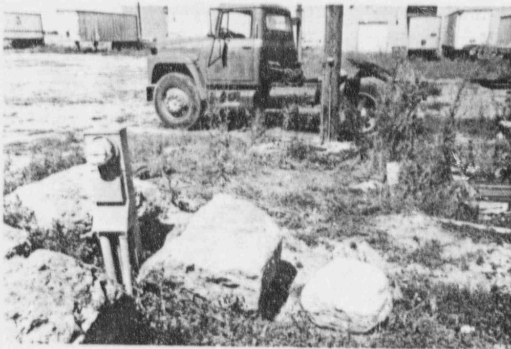
Electric Meter and Power Pole Looking North
