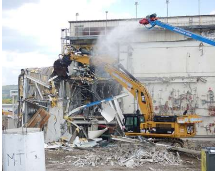
Dust Suppression Equipment Previously Used At WVDP
