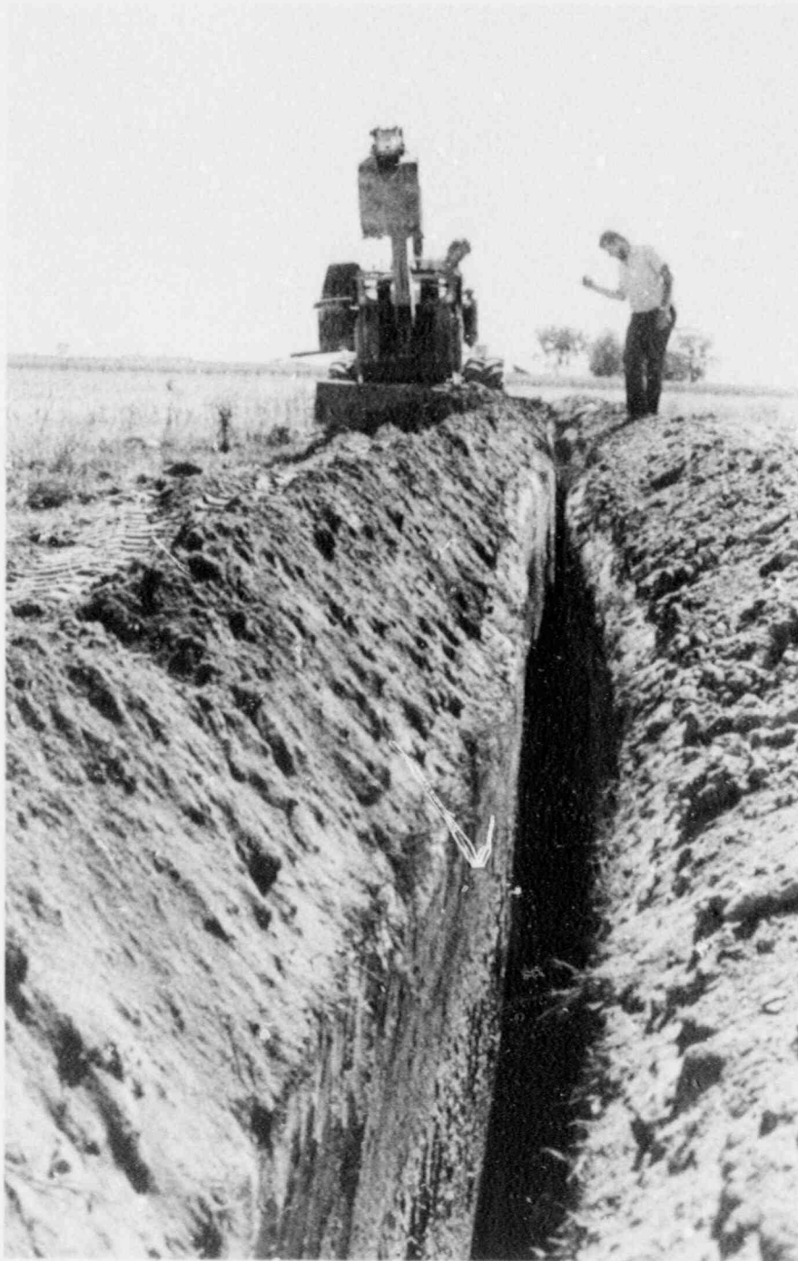
Pictured above is the installation of a horizontal loop for a ground-source heat pump. Piping is installed in trenches at depths of three and five feet.
