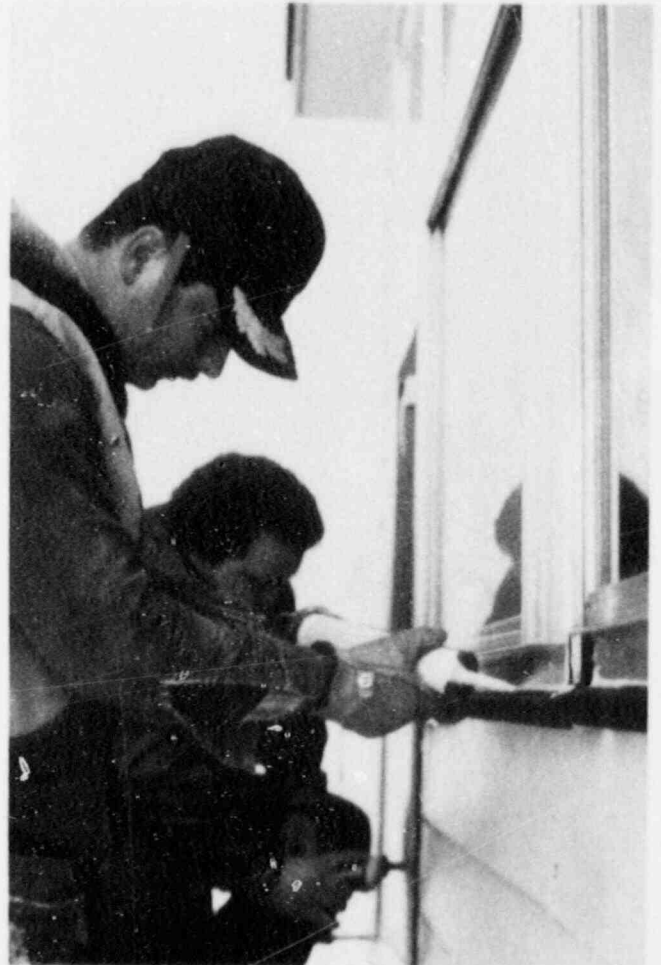
Jeff Morgan, left, and Craig Scroggins from the Bethalto Jaycees caulked windows at the home of a widow. This was funded with part of a $23,000 grant from the Energy Assistance Foundation. The Jaycees completed their three-year project in September 1987, weatherizing 34 homes.
