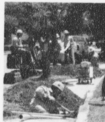
To ensure service reliability, CPS is replacing underground electric cables throughout San Antonio.
