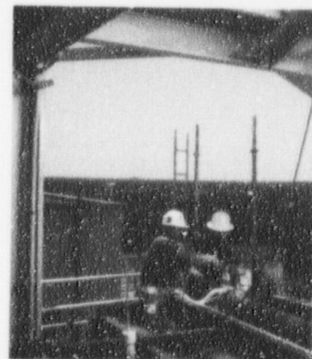
Technicians from the General Maintenance Group prepare a power plant unit to handle the heavy summer load.
