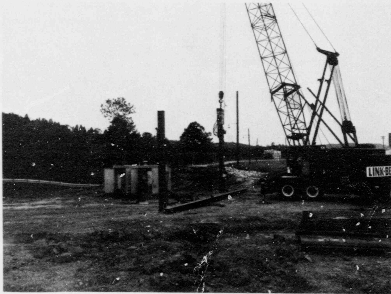
Fig. 11.4. View of barge slip site showing the driving of sheet piling for head wall.
