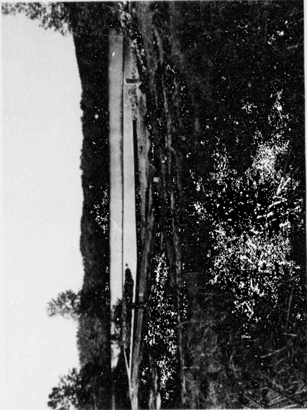
Fig. 11.3. View of barge slip site showing installed silt screen and retaining wall.
