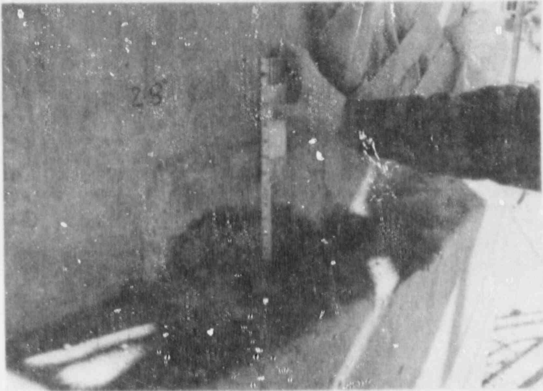
Figure 34. Concrete Void in First Cylinder Wall Lift.
