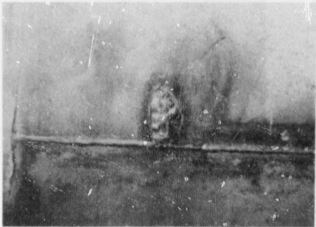
Figure 33. Repaired Liner Flaw.
