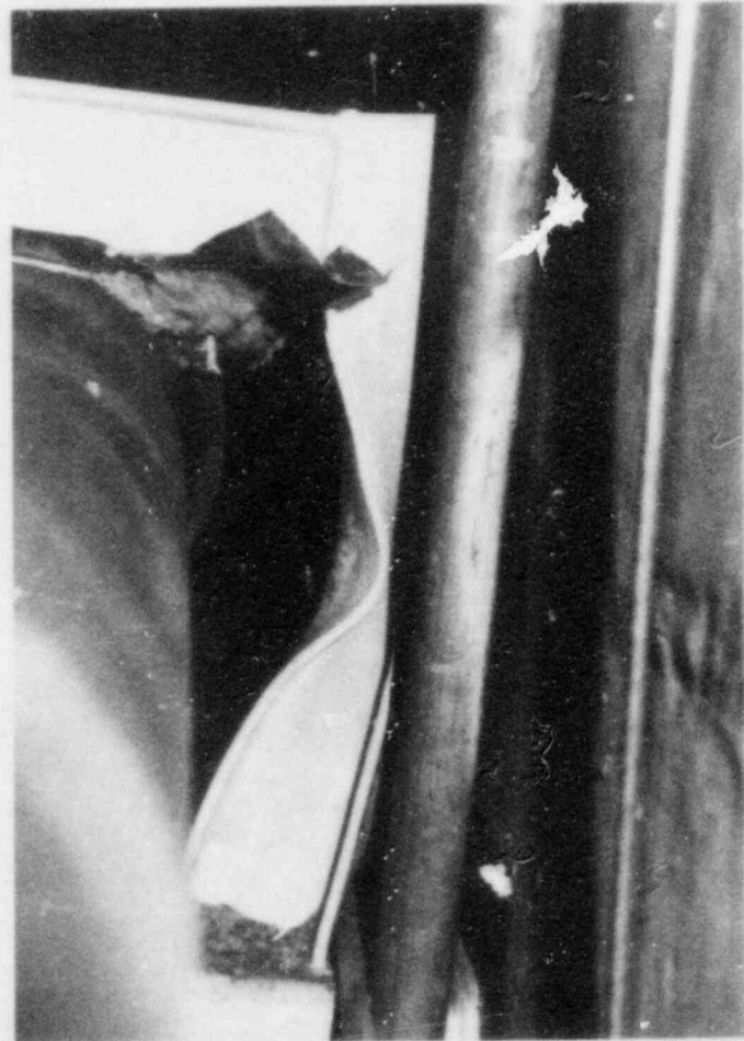
VIEW LOOKING SOUTH ALONG PIPE, DAMAGE DUE TO PIPE LATERAL (WESTWARD) MOTION INDUCED BY WATER HAMMER
