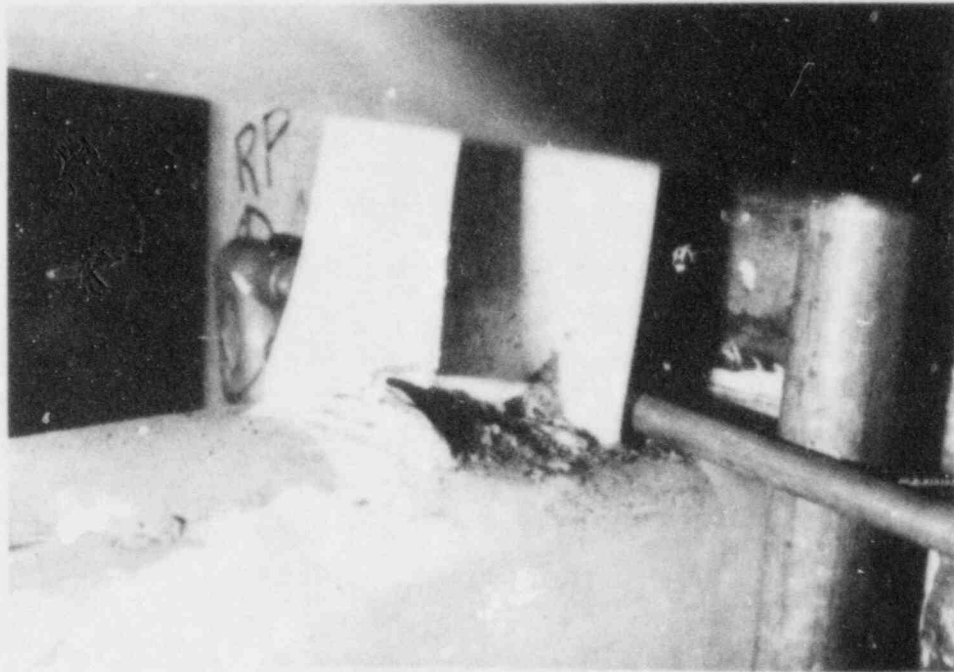
Figure 6.24 Torn Pipe Support Structure HOOK
