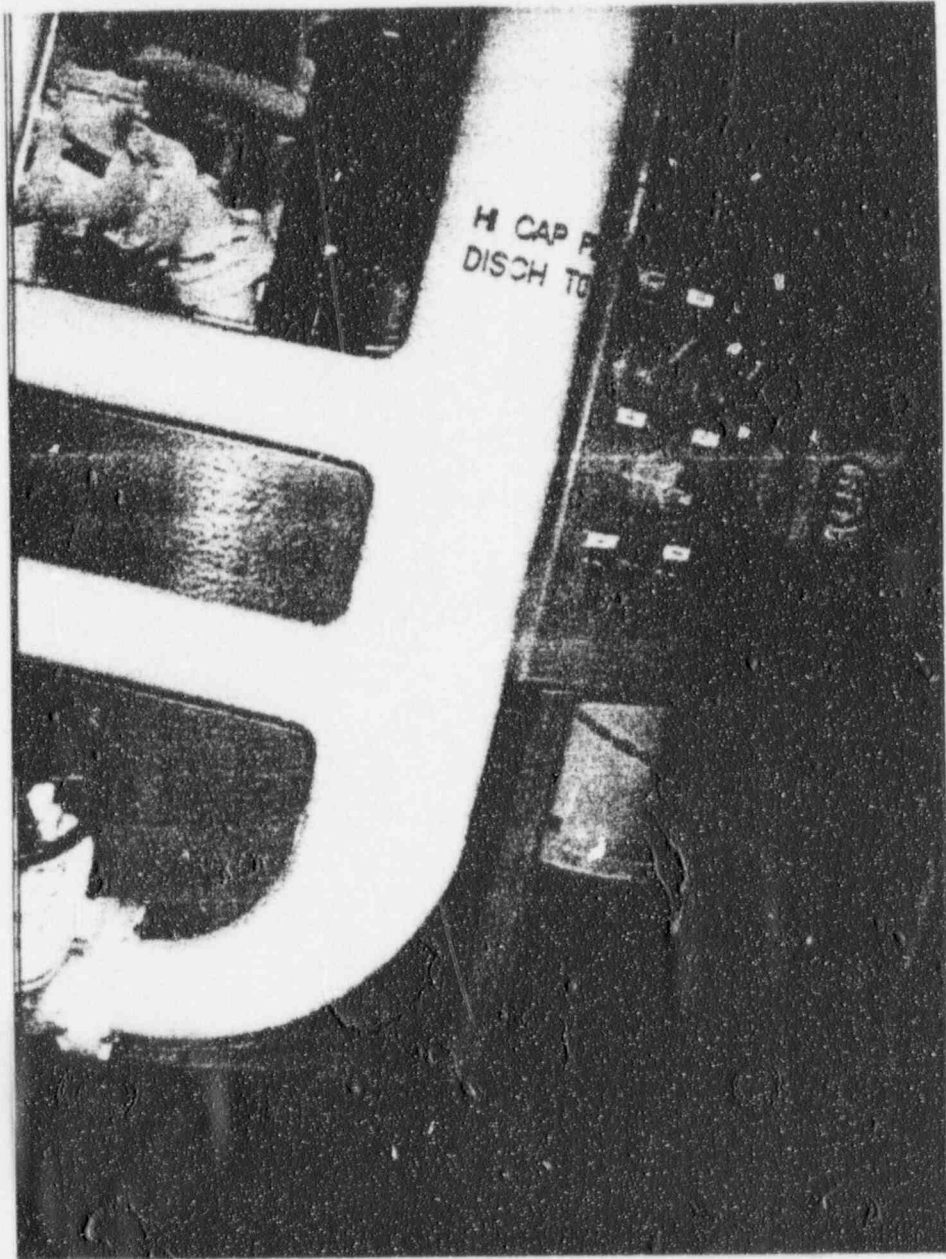
SEWAGE TANK - UNIT 1 TURBINE BUILDING LOCATED IN BASEMENT BESIDES STAIRS NOT ANCHORED TO FLOOR
