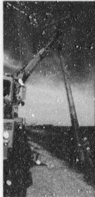
Corn Belt Power's strong transmission system experienced yet another year of delivering a reliable power supply to its member cooperatives, with year-end statistics showing Corn Belt was on line to its members 99.99% of the time during 1996.
