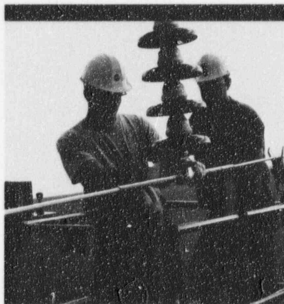
1996 was an important year for new construction of Corn Belt lines and substations, built to strengthen reliability of service to member cooperatives both today and in the years ahead.
