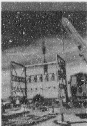
Corn Belt Power Cooperative crews built four substations during 1996 to increase reliability and accommodate load growth in member systems' service territories.
