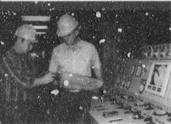
The new combustion control system at Wisdom Station will result in improved plant efficiency, increased plant availability and lower generating costs.
