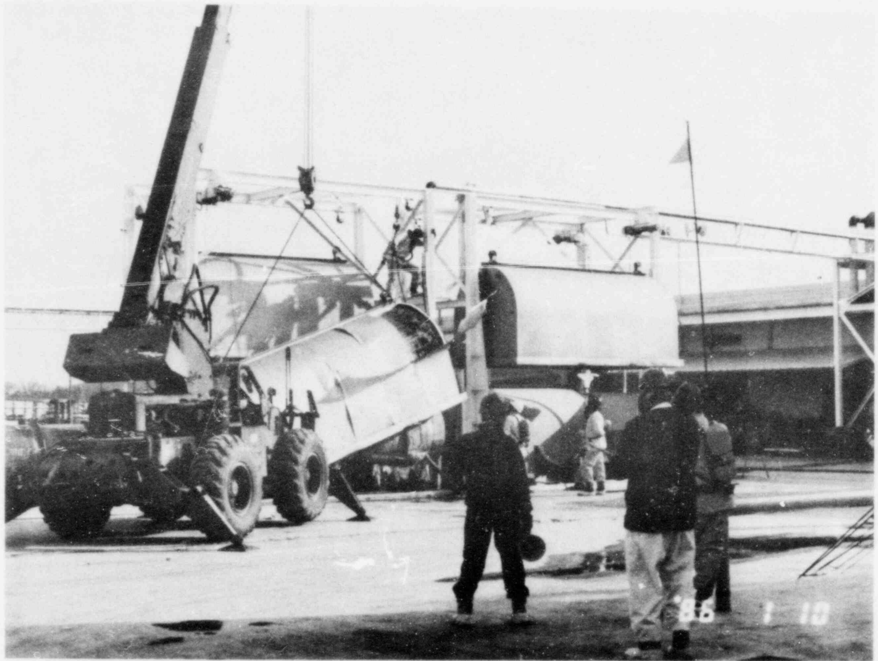
Figure 3.1.1.3A Removing the Steam Chest from the Ruptured Cylinder
