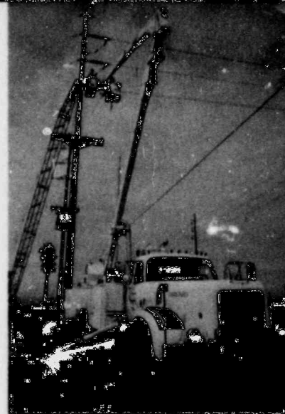
Power construction and maintenance workers installed about 130 miles of overhead electric distribution lines.
