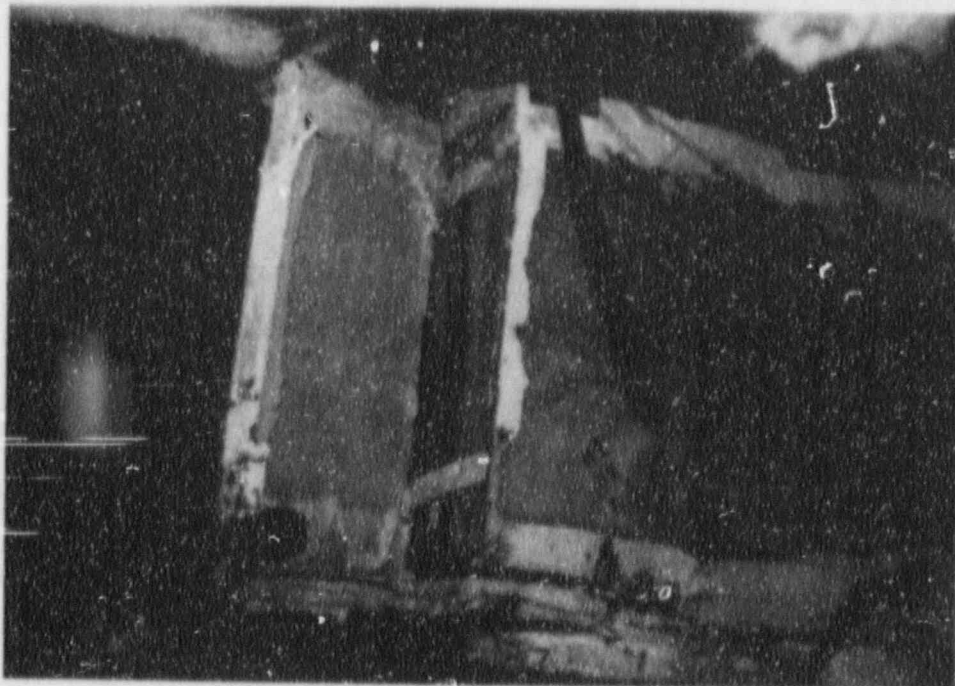
Inner layer removed from front surface of vertical junction box.
