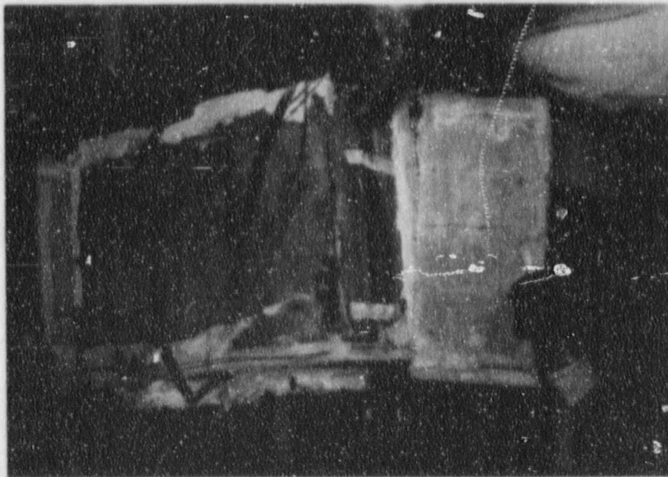
Inner layer removed from right and rear surfaces of vertical junction box.
