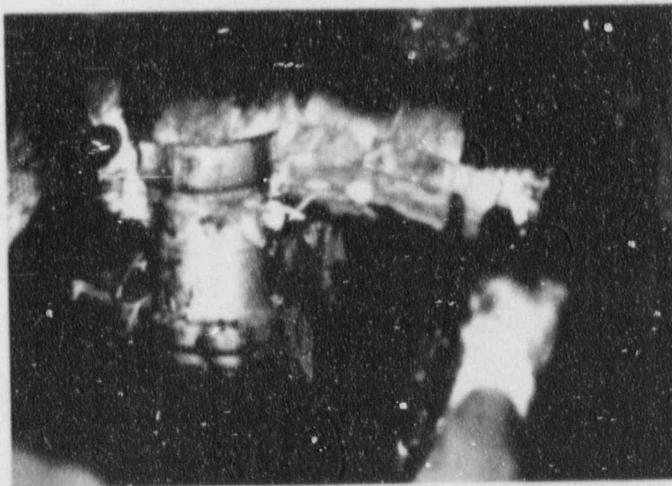
Overlay collar at conduit exit point on right front conduit.
