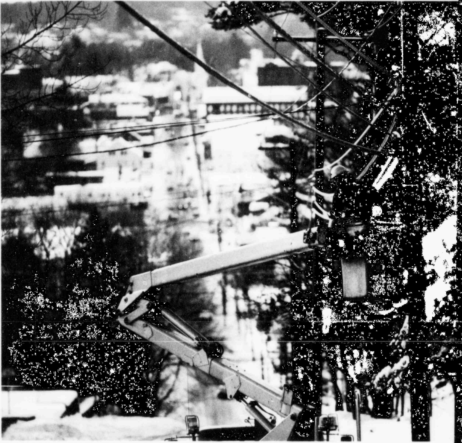
Trudlemann Thomas lattersall prepares to energize a transformer in Milford, Massachusetts.
