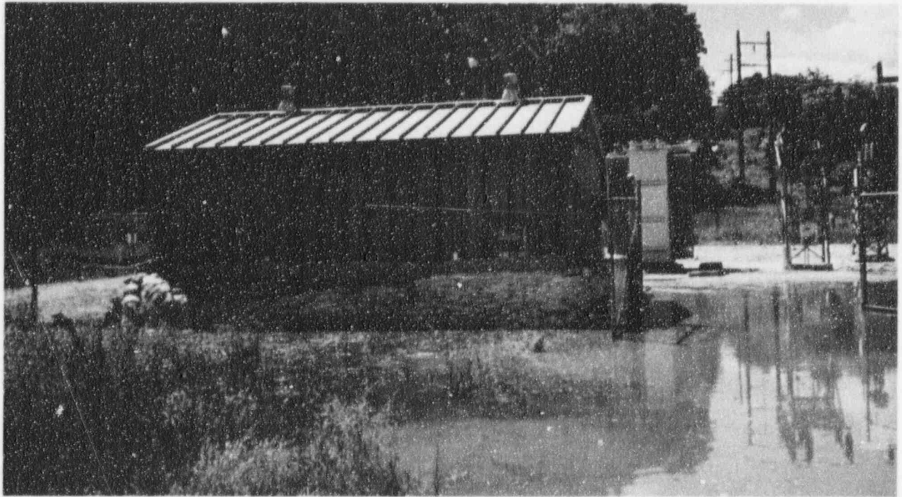
Severe spring flooding again took its toll on rural Illinois as evidenced at this substation near Kampsville. The water was to rise another two feet shortly after this photograph was taken in early June.
