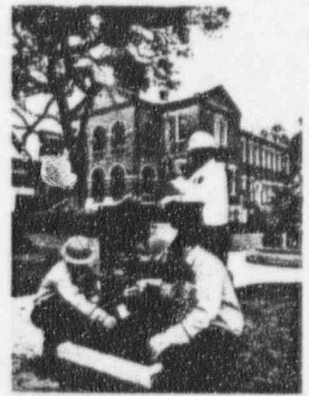
On the Cover: A KUA line crew installs a pad-mounted transformer in front of the historic Osceola County Courthouse in downtown Kissimmee.
