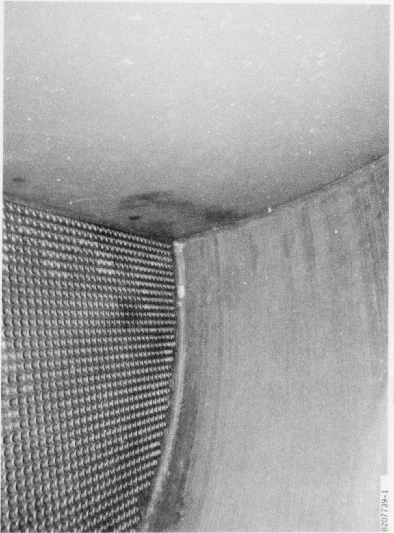
FIGURE 4-11. Hot Leg Surfaces After the NP/LOMI Process
