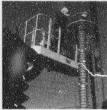
NSP's Chisago substation is one of several in the United States and Canada newly equipped with technologically advanced electrical devices as part of a project upgrading NSP's 500-kilovolt transmission line to Canada.
