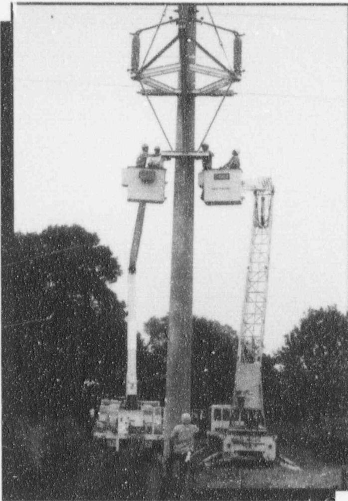
SMEPA'S CREWS INSTALL THE EAST WHITFIELD GOAB SWITCH, WHICH WILL SERVE A NEW SUBSTATION FOR SOUTHERN PINE ELECTRIC POWER ASSOCIATION.
