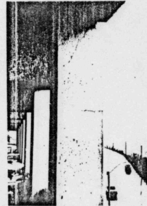
FIG. 1.6.—Inclined Crack in Beam-Column Joint
