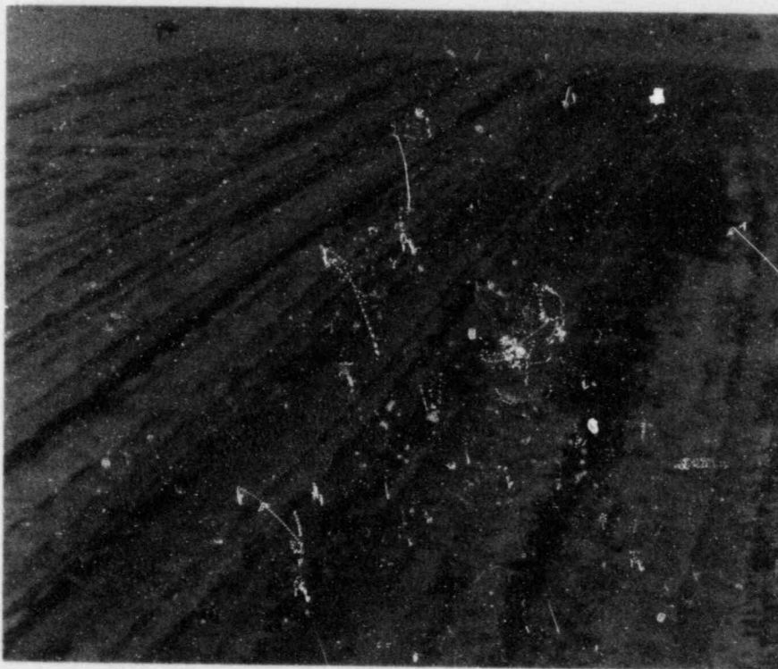
FIGURE 2. Deterioration of the Stabilized Tailings Surface Initially Treated with Retain After Nine Months of Weathering
