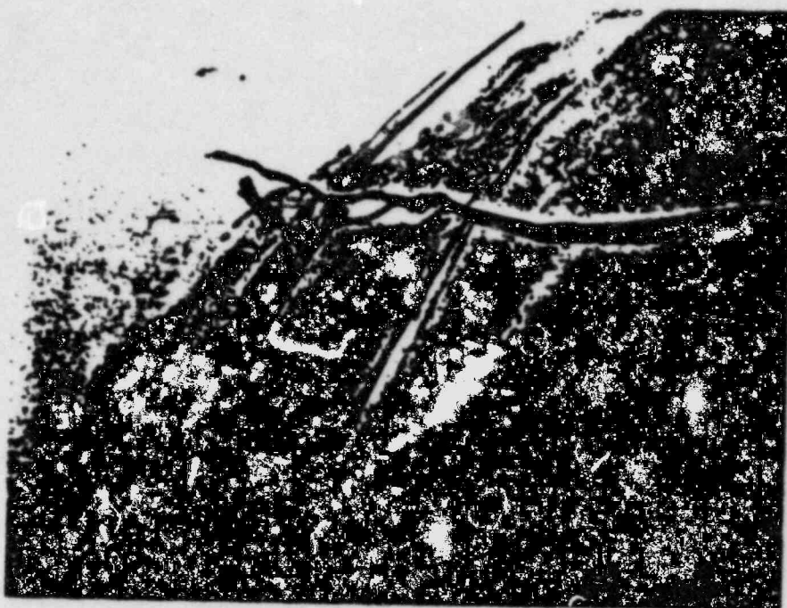
CENTERING PAD CRACKS
