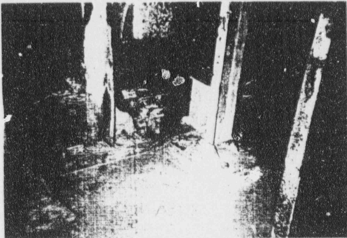
Degradation of Base/Foundation and Corrosion of Steel Supports (B-21)
