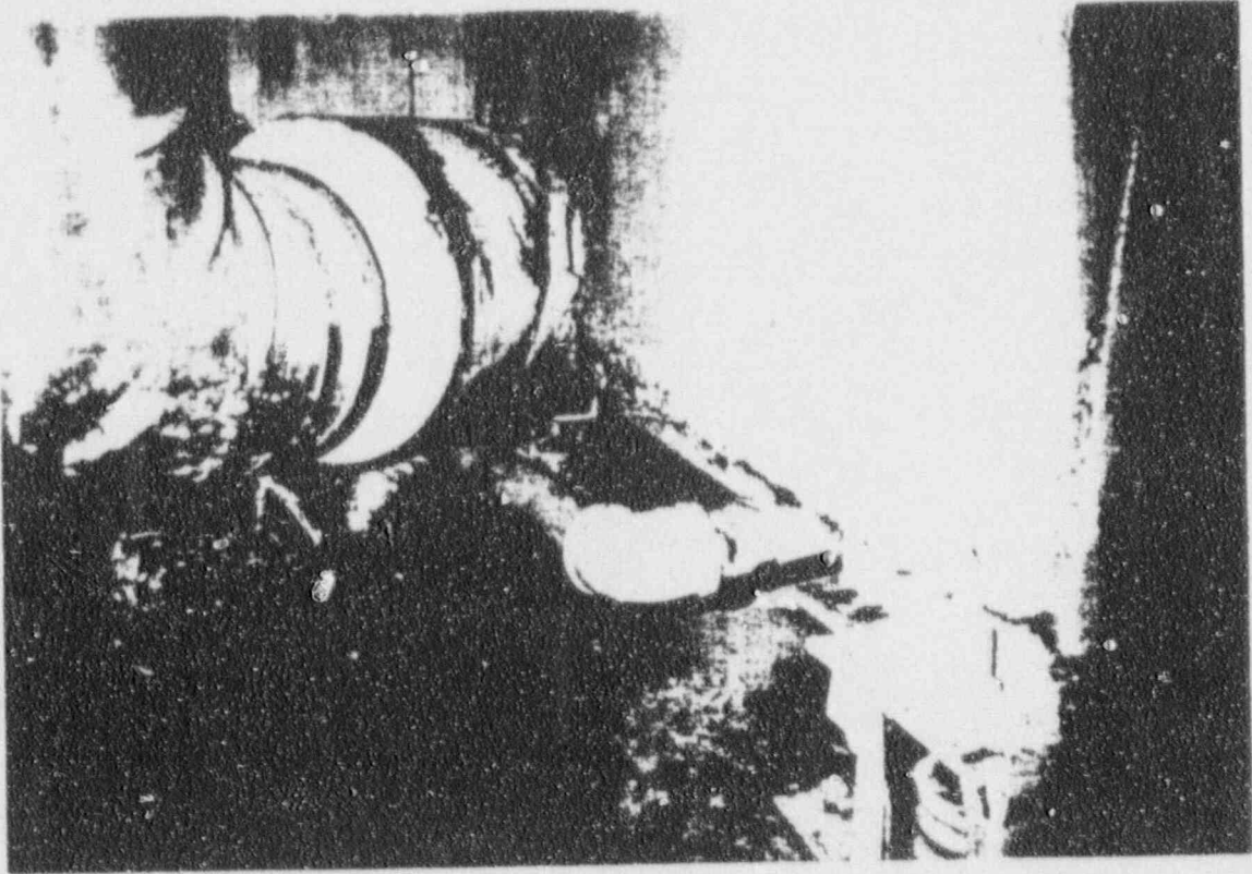
Corrosion of Base/Steel Supports of the Fan Coil Unit (C-3)
