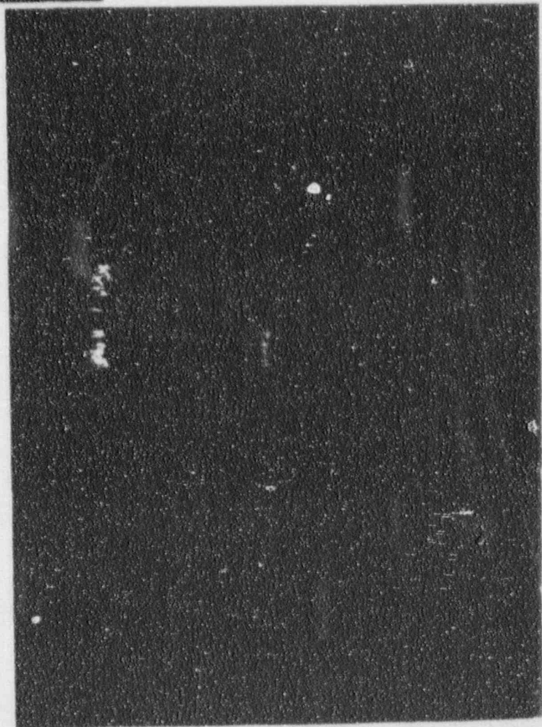
Steam Generator Drain Tank - Cracks, Water Infiltration and Calcium Formation (A-22)
