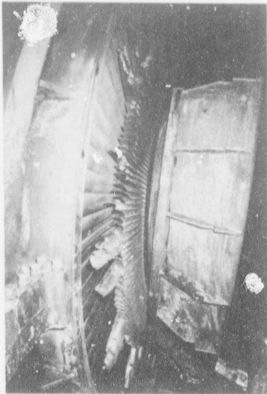
Figure 2. Low pressure turbine Salem Unit 2.
