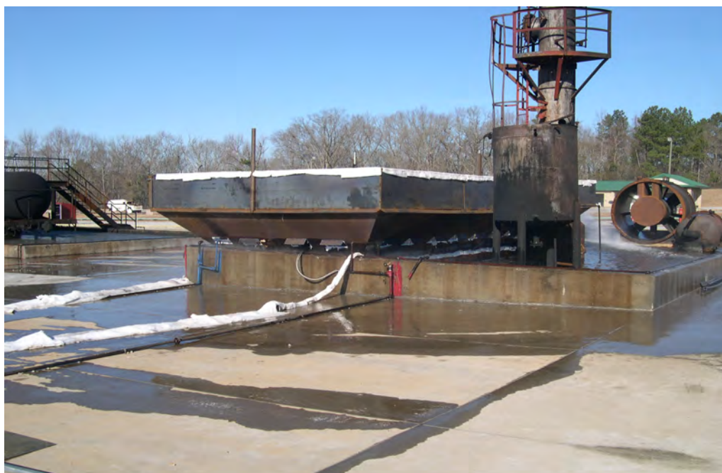
Figure 3-33 Test Setup with Steel Diffuser Plates
