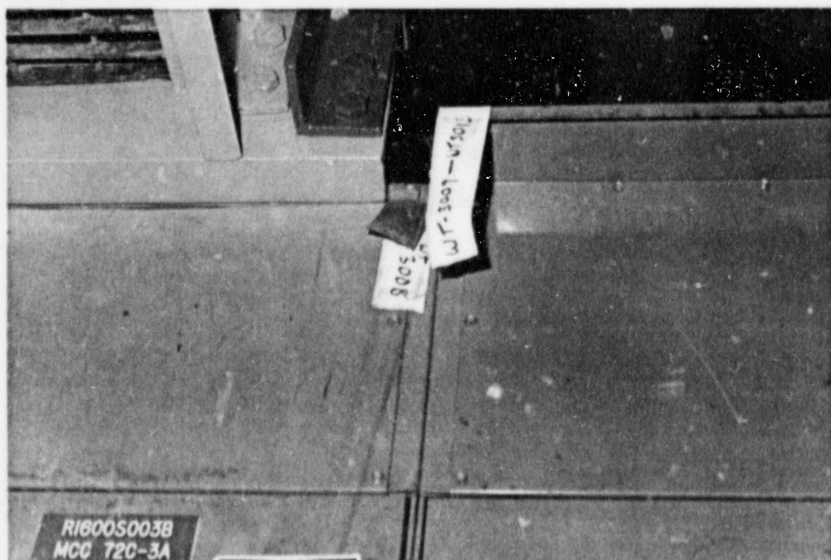
Photograph 3.10.1 MCC 72C-3A with EECW piping overhead and stair landing in direct contact.
