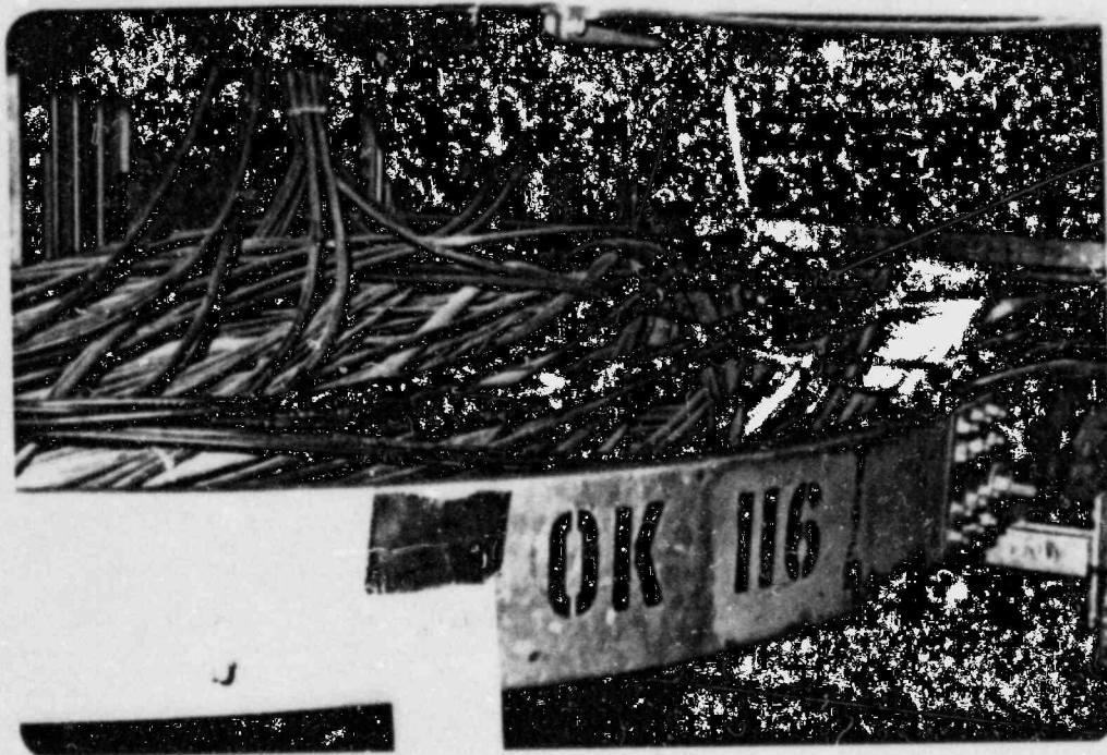
Photograph 3.11.3 Example of cable tray overfill.
