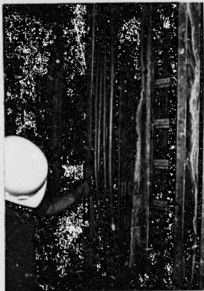
Photograph 3.11.2 Cables installed in vertical tray-cables not attached to tray.
