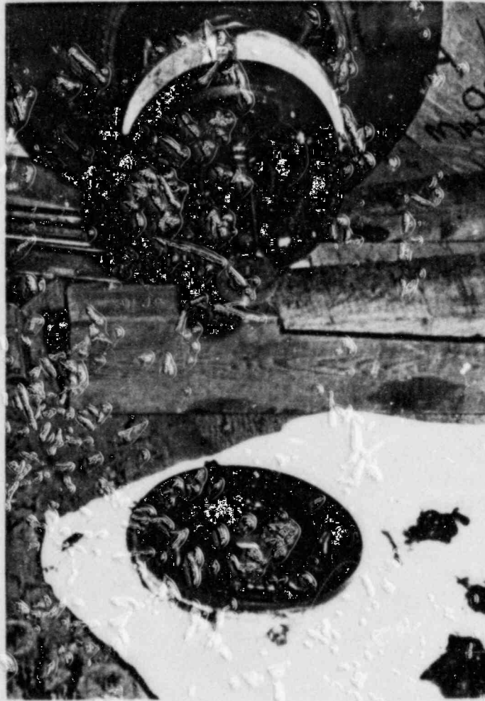
Photograph 3.7.4 EECW Pump (Div. II)-Pump Disassembly. Inside of pump bearing housing shown. No evidence of corrosion or damage. Bearings in very good overall condition.
