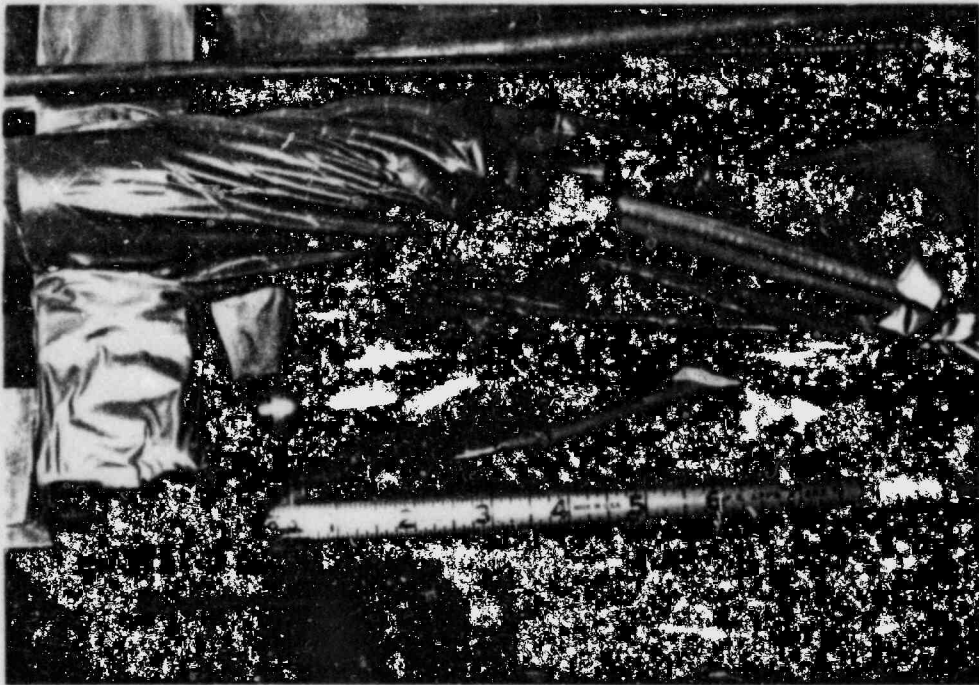
Photograph 3.13.1 Example of radiation monitor cable disconnection at sensor.
