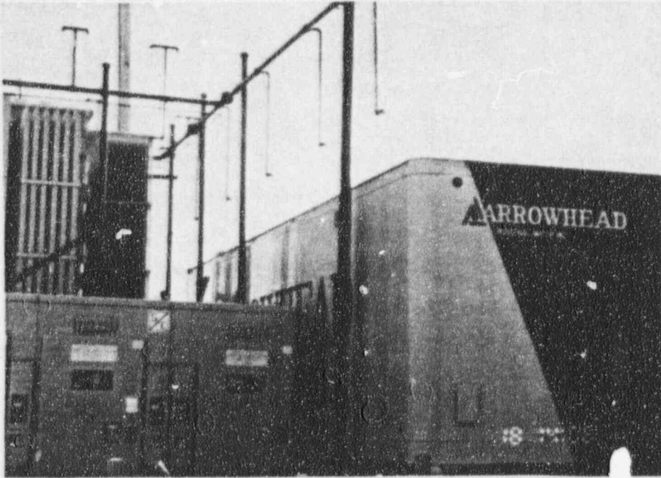
Figure 5: Unanchored Industrial Water Van in Close Proximity to the SBO Transformer Fire Suppression Distribution Piping and System Support
