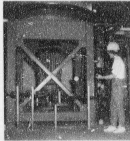
During 1991, Advanced Separation Technologies sold seven ion Separation (ISEP) machines, including this installation at Great Lakes Sugar near Toledo, Ohio.
