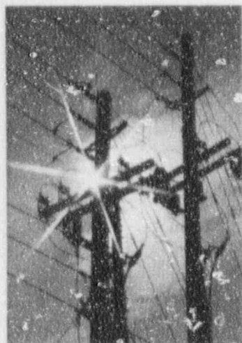
Miles of transmission lines help KUA provide reliable electric service.
