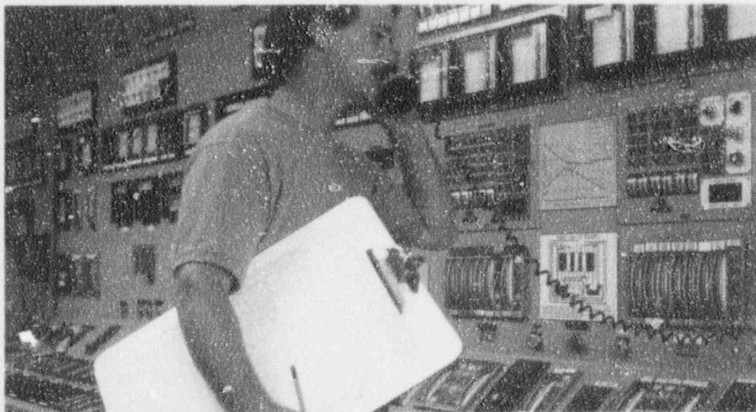
Deerhaven Generating Station's control room is at the center of the state's electric facilities.
