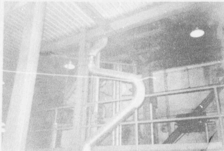
Figure E.55 Expansion Loop on Support of Small Bore Hot Line in Glendale Unit 3
