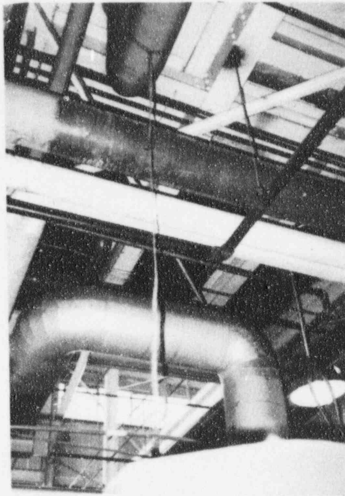
Figure E.67 Field Fabricated Hangers in Olive Unit 2
