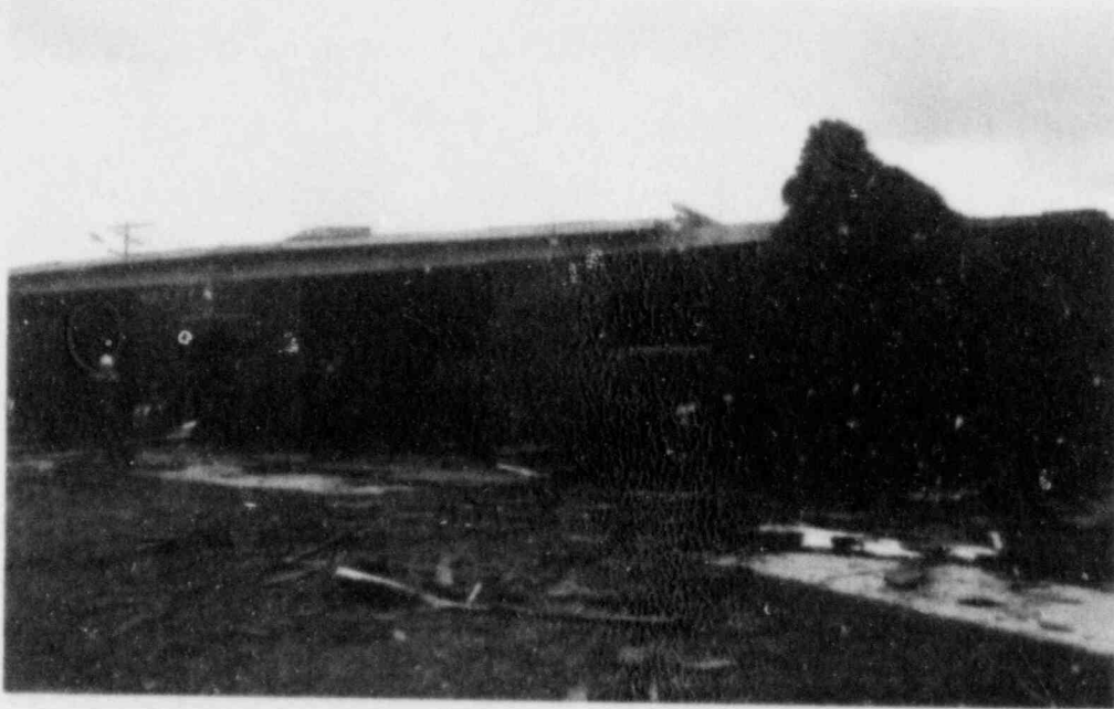
FIGURE 12. ROOF DAMAGE TO RECREATION BUILDING (damage was confined to roof fascia and roof corner).
