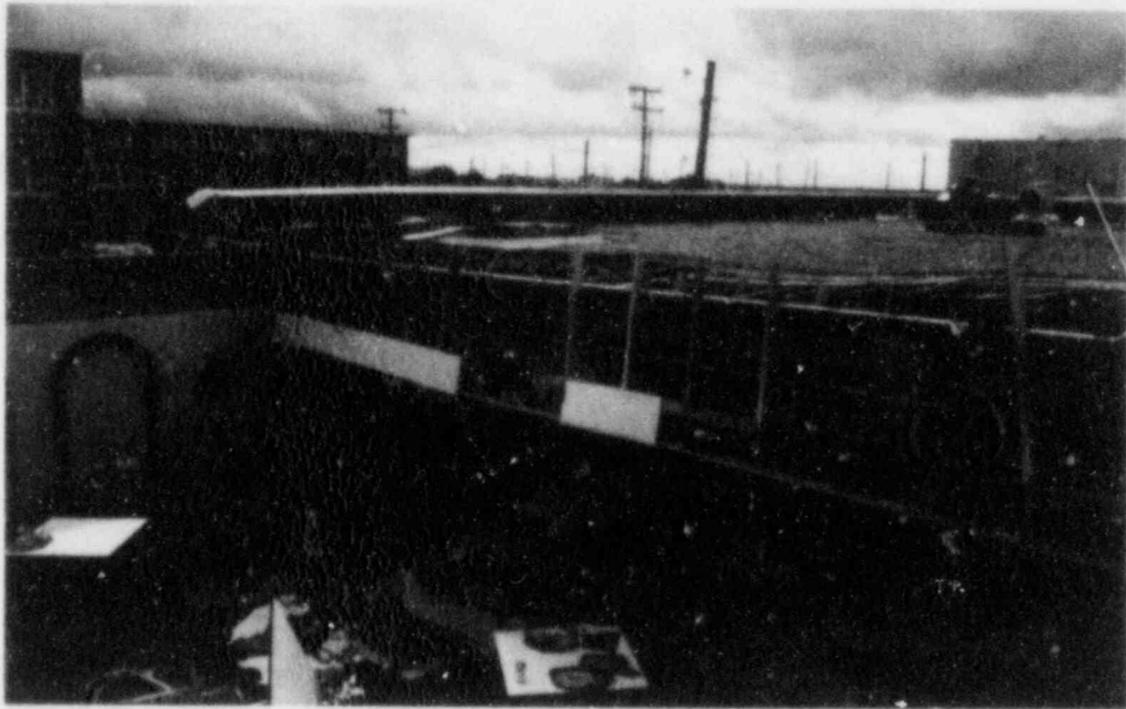
FIGURE 11. DAMAGE TO THE DINING HALL CAFETERIA ROOF.
