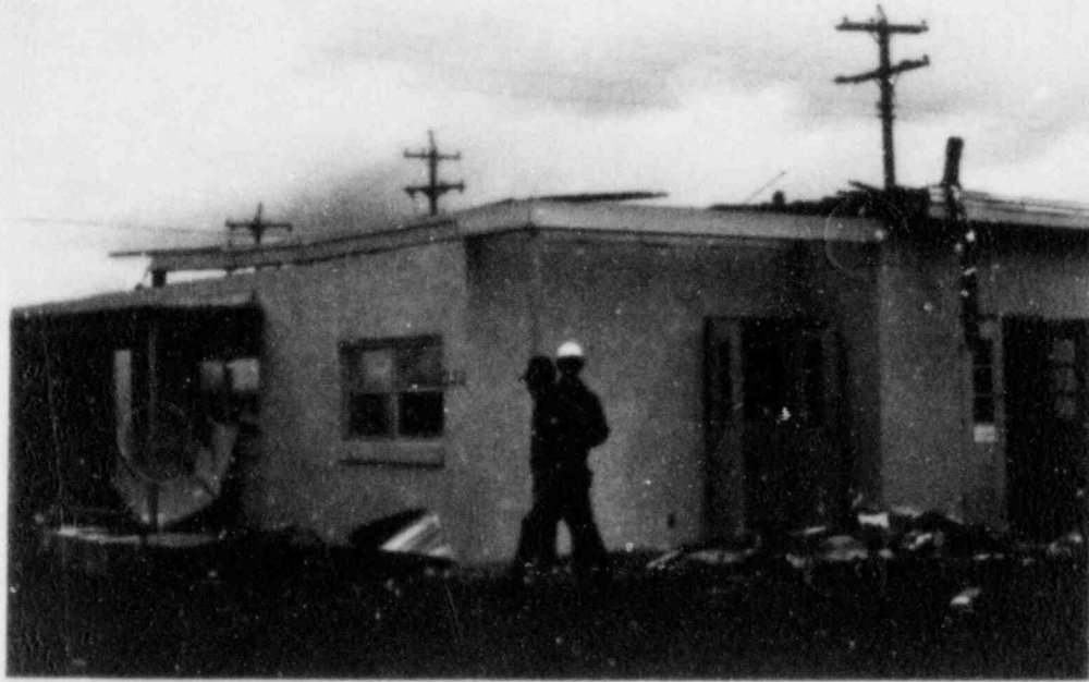
FIGURE 6. VIEW OF SOUTHEAST CORNER OF VETERINARY CLINIC (the cracks in the mortar joint below the bond beam occurred as the roof lifted).
