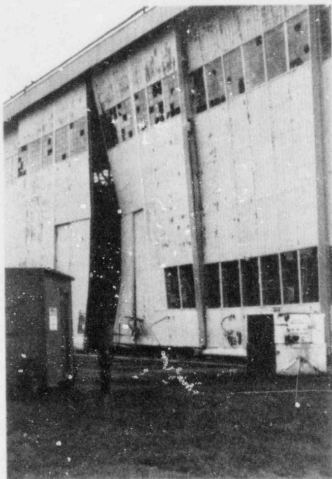
FIGURE 15. DOORS OF AIRCRAFT HANGAR (force of wind bent doors inward).
