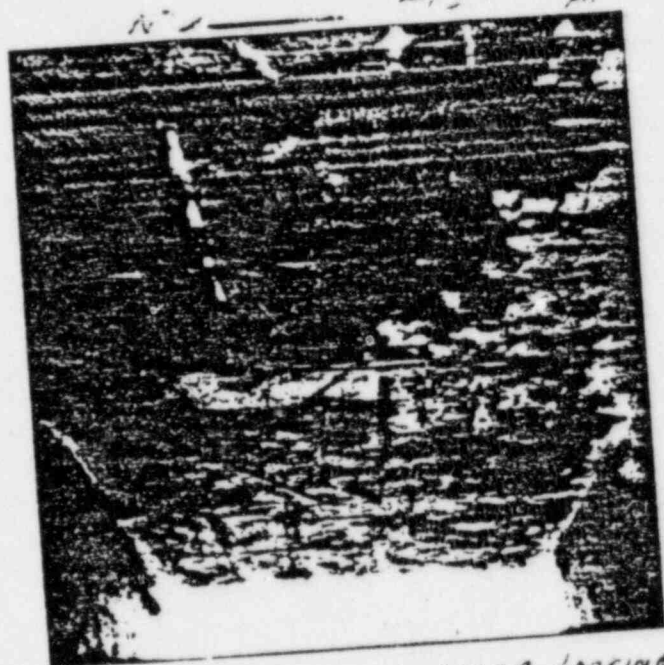
7/2/83 NORTH BAY UNDERSLAB LOCKING EAST. CUT GROOVE PATTERNS VISIBLE
