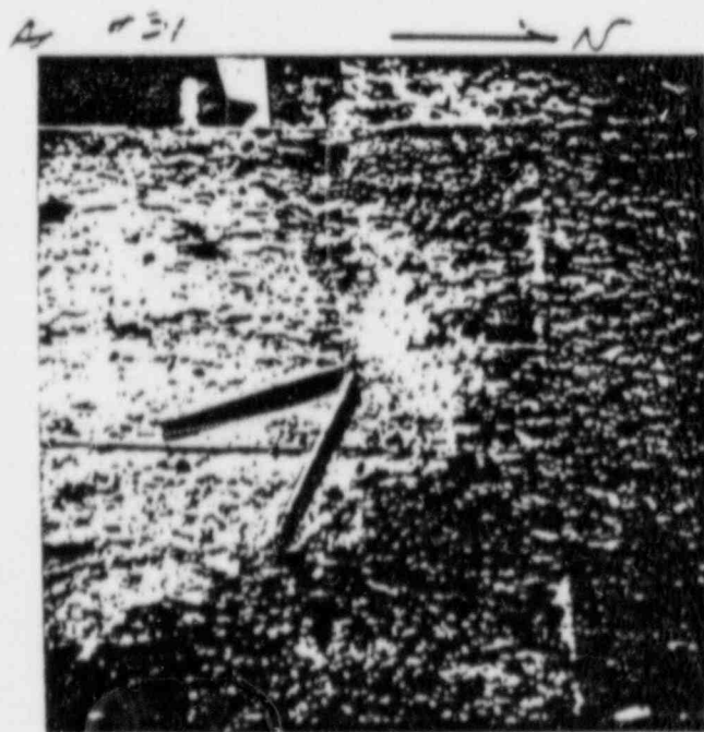
7/11/83 RATE No. 5B (NORTH WEST CORNER) APPEARANT LOSS ON CONTACT AREA 211" x 6". THE M.B. APPEAR TO HAVE SLIPPED ON THE WEST SIDE (1 1/2" TO 2" GROUND IN)
