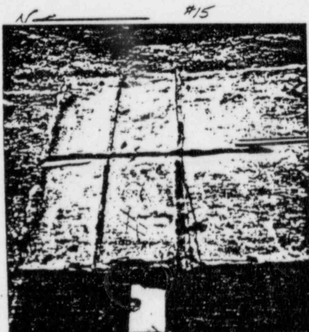
6/29/83 RATE No. 2 (NORTH END) CONCRETE CUT "H" PATTERN LEAD WOOL/EXP. METAL BULKHEAD 4 GROSS NIPPLES FOR WOOD RATE
