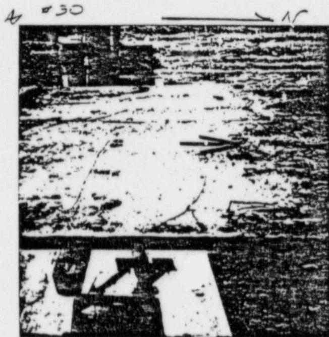
7/11/83 RATE No 5B (NORTH END) 3 RD DRYPACK TEST RATE BUT MADE WITH SAND/CEMENT MIX #713
