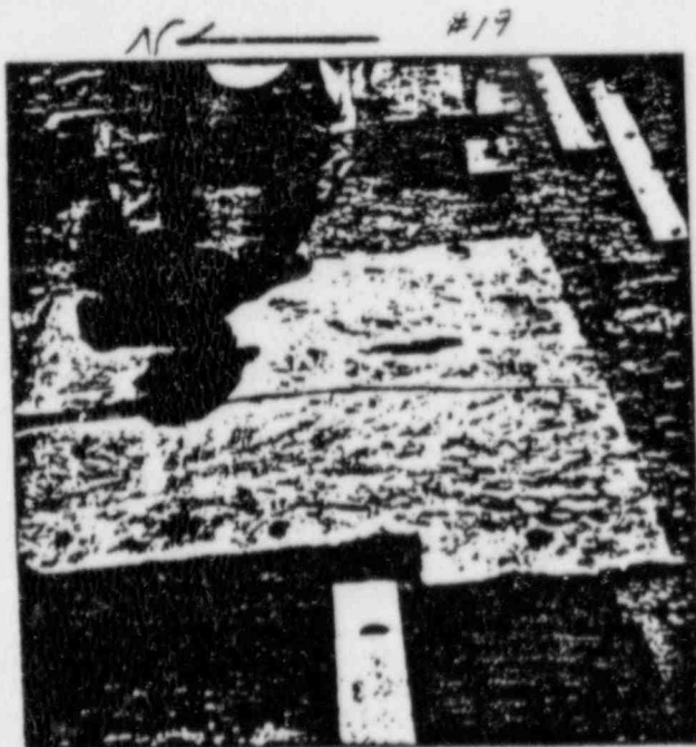
6/29/83 PLATE No. 4 (SOUTH END) NO CONCRETE CUT, 4 NIPPLES FOR RATE, WOOD BULKHEAD
