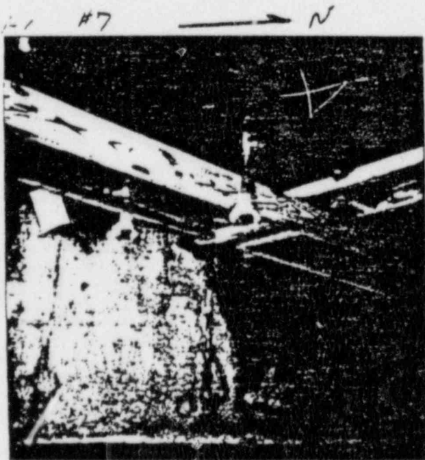
6/28/83 TYPICAL GIRTS NIPPLE SET-UP WITH C.P. COUPLING, PIPE NIPPLE, VALVE AND WELDED NIPPLE. (SAWING @ RATE No. 4)
