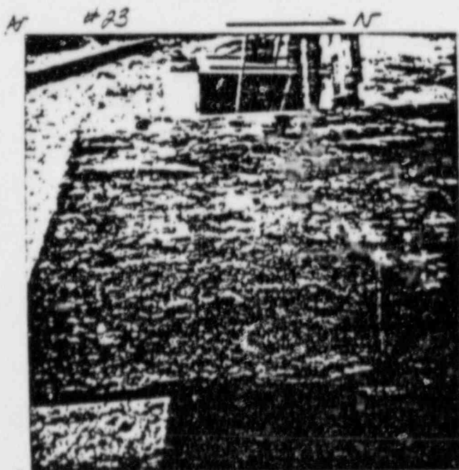
7/12/83 RATE No. 5A (SOUTH END) SECOND DRYPACK TEST RATE AT SAME LOCATION ALSO USING MASTERFLOW #713
