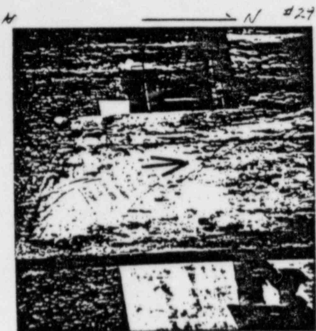
7/7/83 RATE No. 5B (SOUTH END) 3 RD DRYPACK TEST RATE BUT MADE WITH SAND/CEMENT MIX #713
