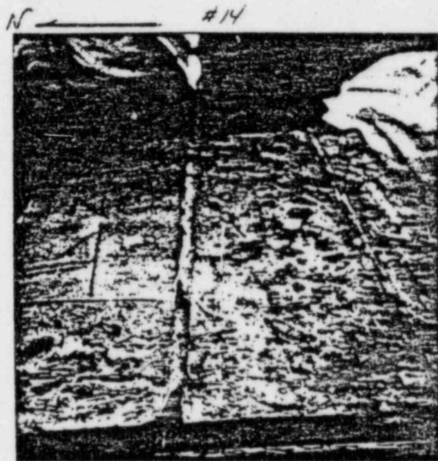
6/29/83 RATE No. 1 (SOUTH END) CONCRETE CUT PARALLEL LINES, 4 NIPPLES FOR RATE, WOOD BULKHEAD
