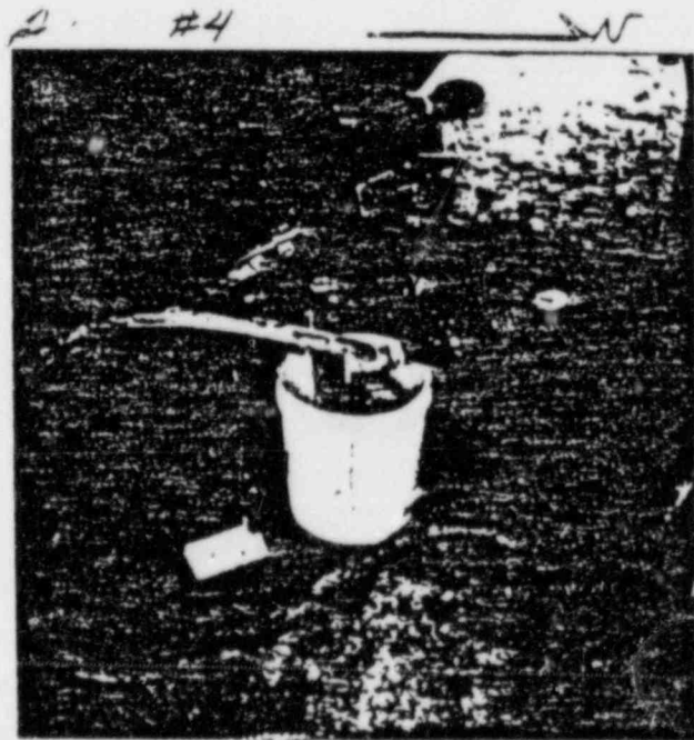
6/28/83 GROUT PUMP SET UP PUMP = AIRPLACO MODEL #HG-5, S.N. - 821121, Pressure Gauge 0-60F 2 1/2" Ø DIAL ALL APPEAR TO BE IN GOOD CONDITION.
