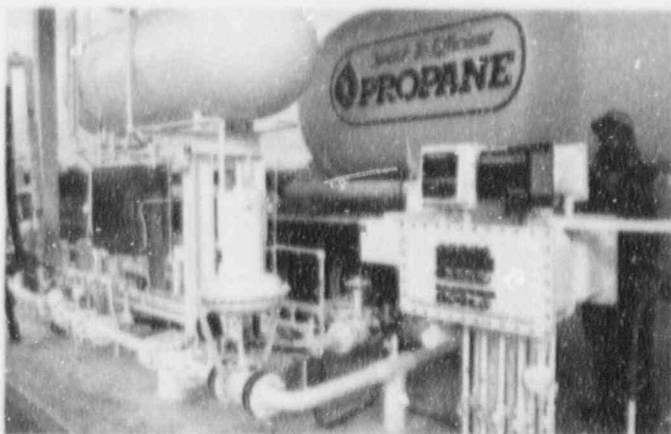
New truck docks were installed at the caverns in 1991. This enhancement doubled the loadout capacity to eight trucks per hour. The average load on each truck is 9,500 gallons.
