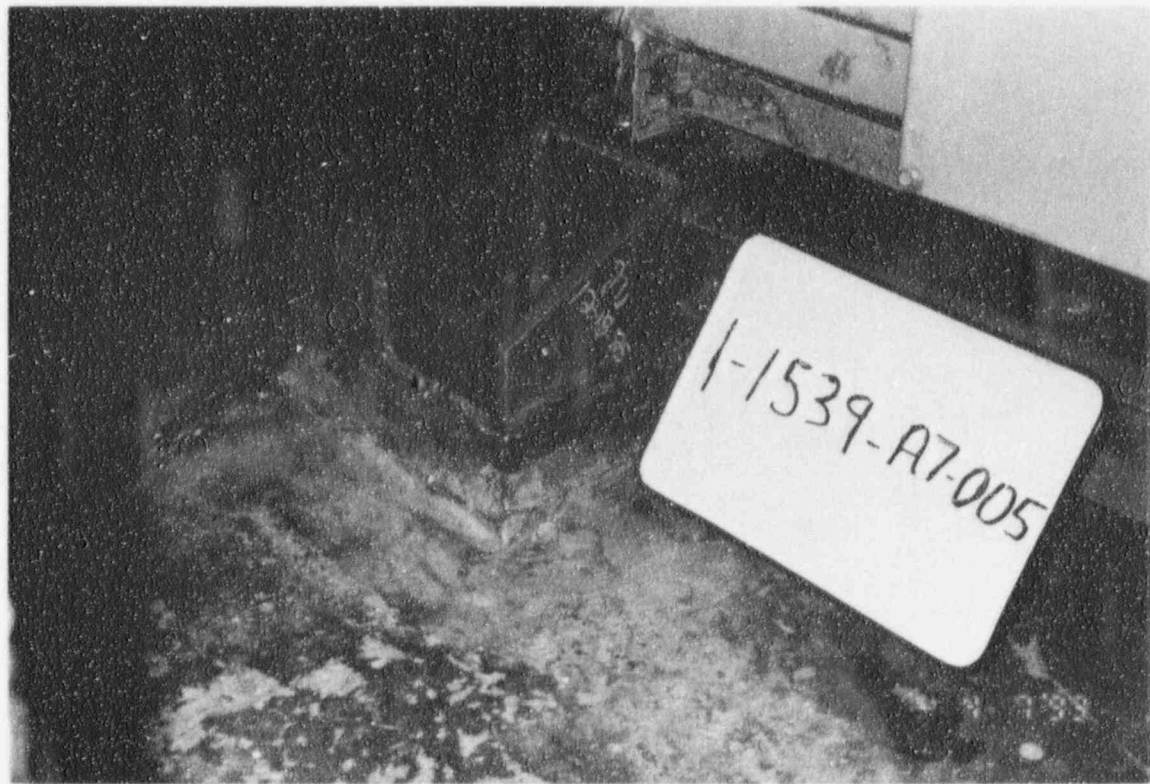
Figures 3.1-50 and 3.1-51 Bolted Anchorage for the Control Bldg. Normal AC Room ESF Air Conditioning Unit (1-1539-A7-005-000)
