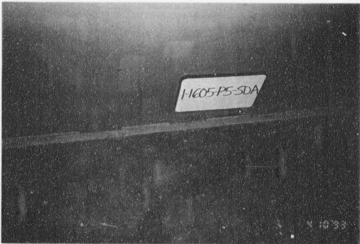
Figures 3.1-54 and 3.1-55 Welded Anchorage of the Shutdown Panel Train A Motor Control Center (1-1605-P5-SDA)
