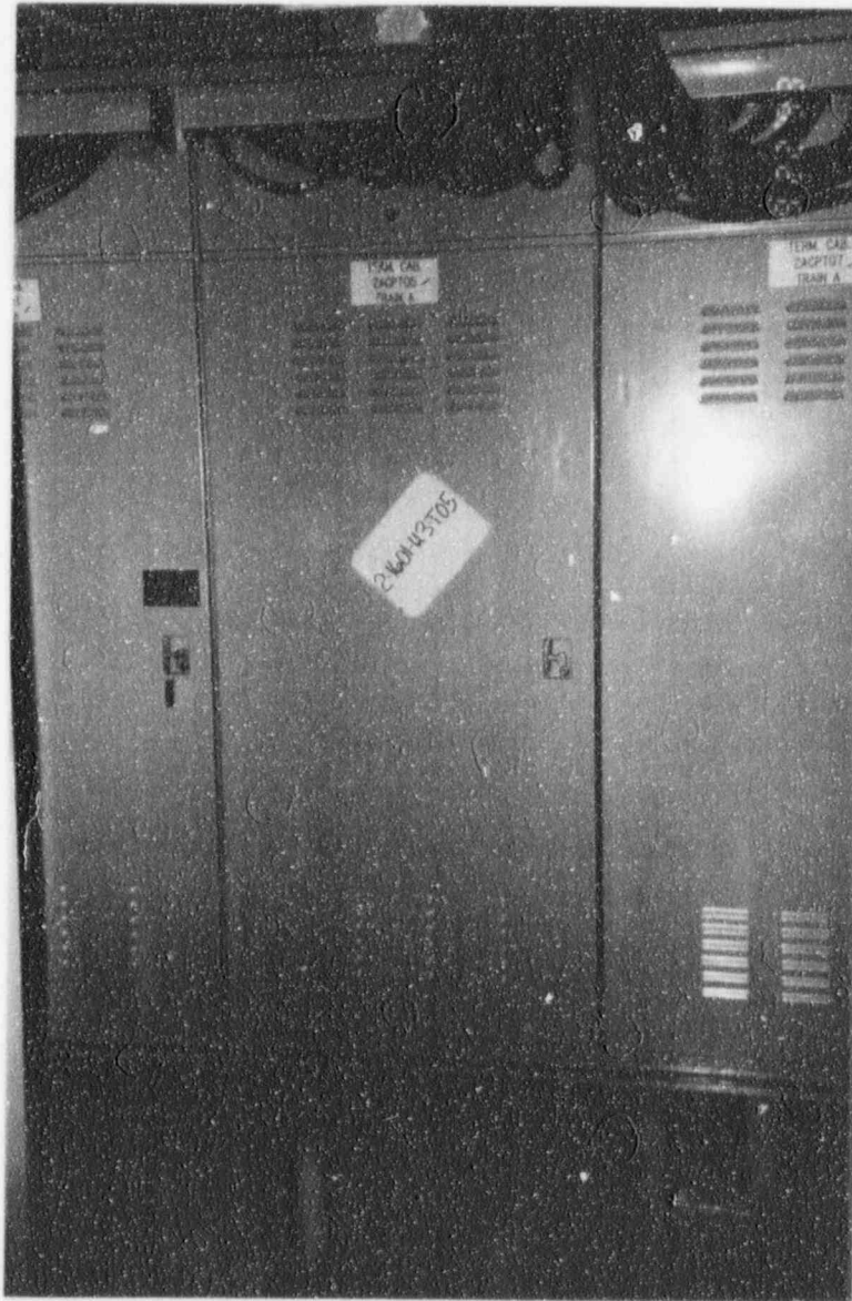
Figure 3.1-58 Welded Anchorage for the Main Control Board Termination Cabinet (2-1601-U3-T05)
