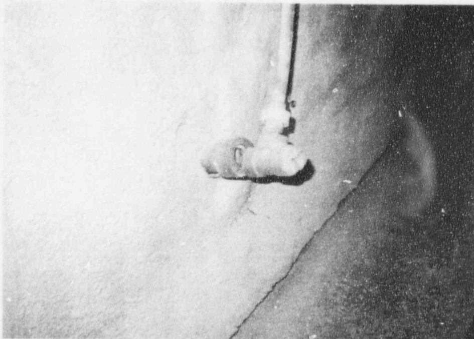
Item 27 - Unit 2 Elev 992 Column H12 Furnace Probe Pipe Broken Off
