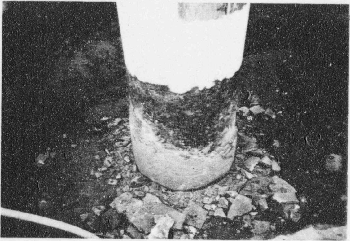
Glendale: Picture 35 (20" Vertical Riser to Cooling Tower Damage)
