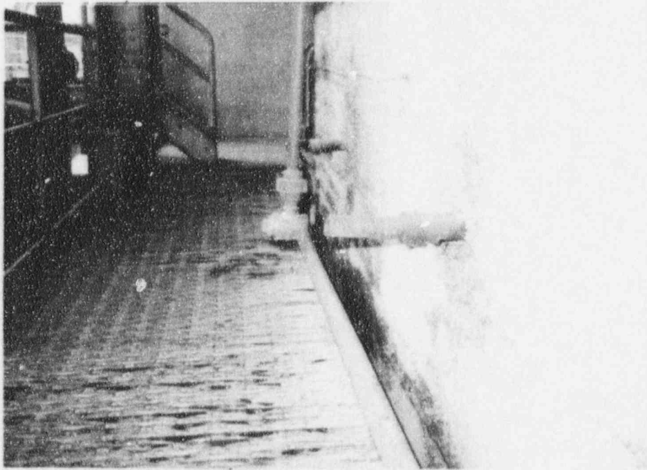
Item 30 - Unit 1 Elev 975 Column J5 Boiler Probe Pipe Broken Off
