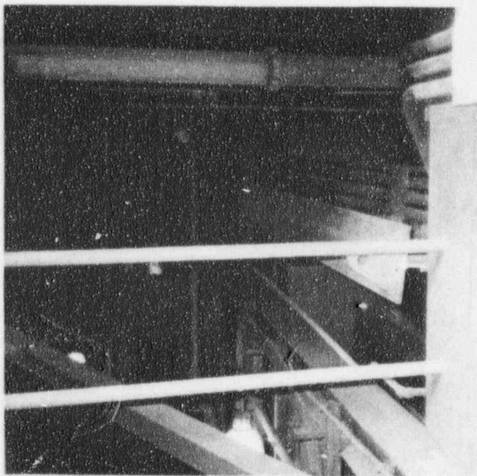
Item 36 - Unit 2 Elev 930 Front Boiler Buckstays Bent - Plate 2
