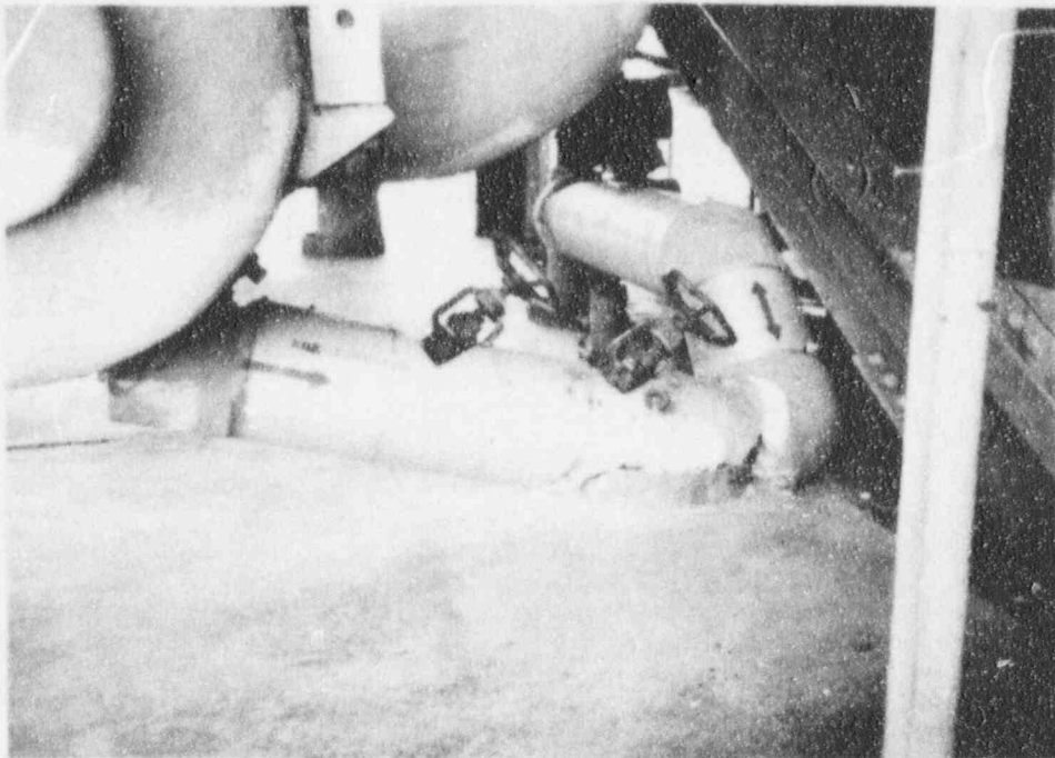
Item 21 - Unit 1 Elev 1006 Main Steam Bottle Drains Damaged
