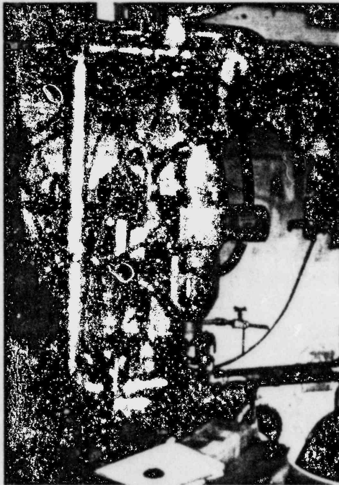
A) TYPICAL MOV IN MSF AREA
