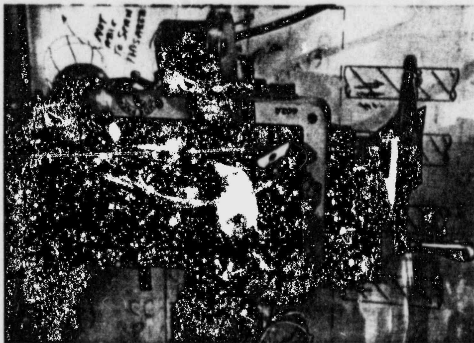
B) MOV PARTIALLY DISASSEMBLED FOR NRC INSPECTION
