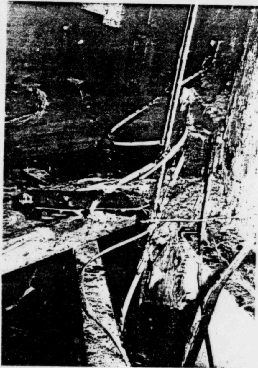
Figure 3.16 Blowdown damage to fiberglass insulation covering the HDR pressure vessel
