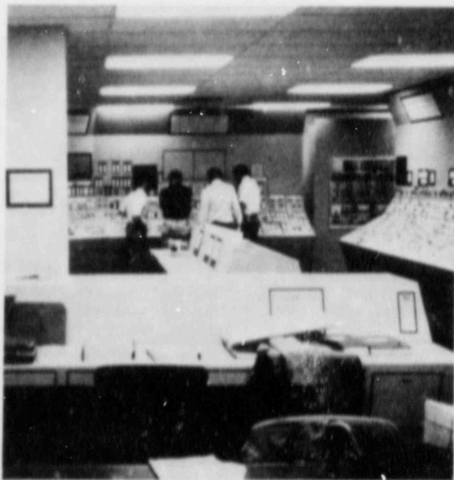
NRC staff concerned with human factors in nuclear power plant operations are shown reviewing a mock-up of the control room for the South Texas plant. Early review of a mock-up reduces the number of changes and associated costs after the actual control panels are fabricated and installed.
