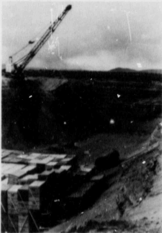
A dragline is used to excavate trench construction access ramp at the Hanford low-level waste disposal site. The horizontal stratigraphy allows the trench walls to hold firm.
