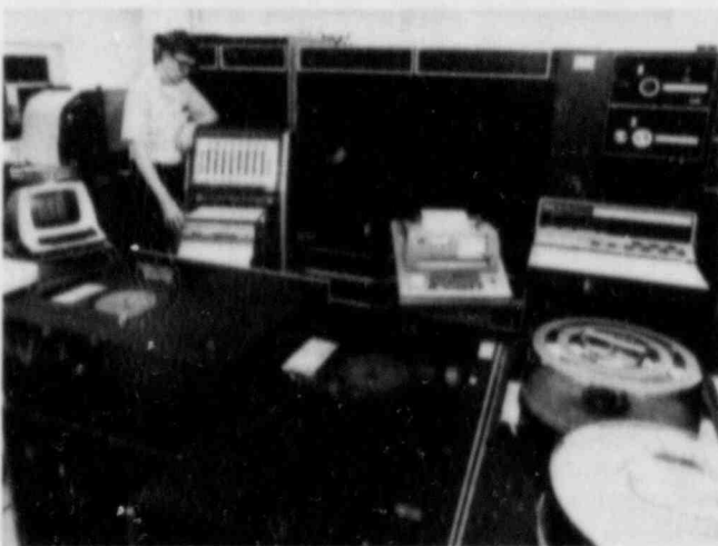
In the photo above, an automated on-line noise surveillance system is demonstrated at the Sequoyah Unit 1 facility in Tennessee. Below is a computer laboratory at the Oak Ridge National Laboratory which is used in the study of plant dynamics and control, as part of NRC research on the safety implications of control systems.
