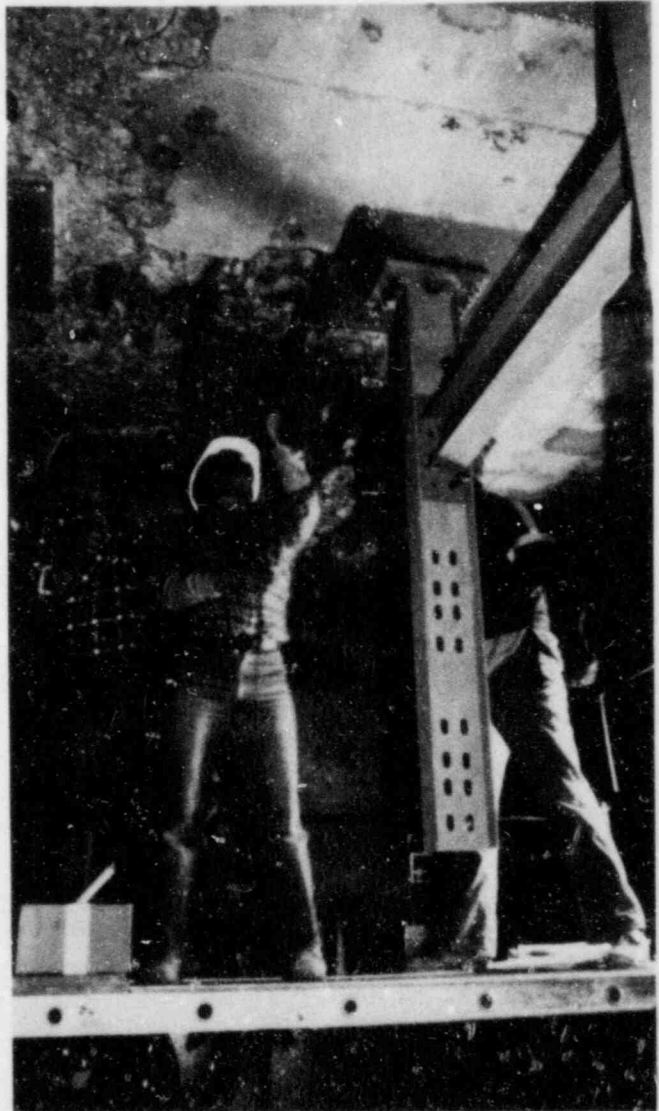
The NRC inspector in the foreground is examining conditions under the spent fuel pool floor at Nine Mile Point Unit 2 in New York. IE Bulletin 82-03 informed licensees that stress corrosion cracking of welds found at the plant led to degradation of recirculation system piping. The phenomenon was judged to have a high degree of safety significance; operating boiling-water reactor plants were required to take preventive and/or corrective action. Among the actions required was a demonstration of the detection capability of ultra-sonic methods for examining welds in the thick-walled recirculation system piping.
