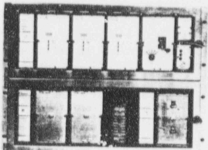
Fig. 4. Two additional input restraint unit TUC 4's (lower left) and lock-out relay MVB 4 (lower right) in a DSE with five input-restraints.
