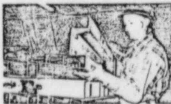
Unique steel lagging, designed by Mergentime, meets NRC requirements for nonorganic, nonbiodegradable materials. Also see cover.
