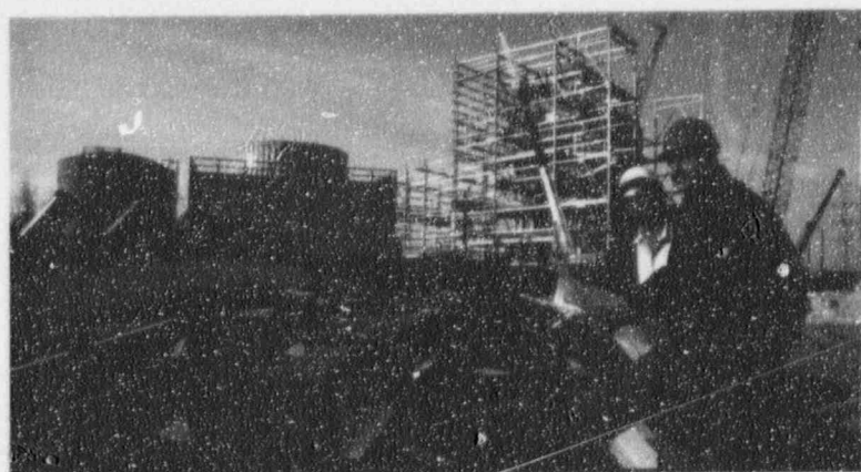
When assembled, conveyers (foreground) will transport tons of tire chips to the combustion facility (right, background) at the Ford Heights Tire-To-Energy Project.
