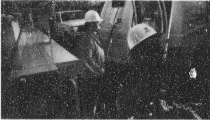
KBLCOM employees prepare to upgrade existing cable with fiber optic technology that will increase capacity and provide the capability for interactive services.
