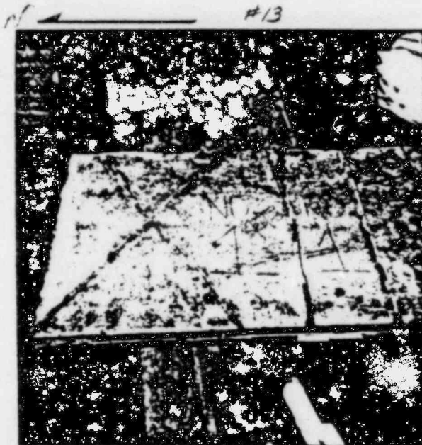
6/29/83 RATE No. 1 (NORTH END) CONCRETE CUT "X" PATTERN, 4 NIPPLES FOR RATE, WOOD BULKHEAD
