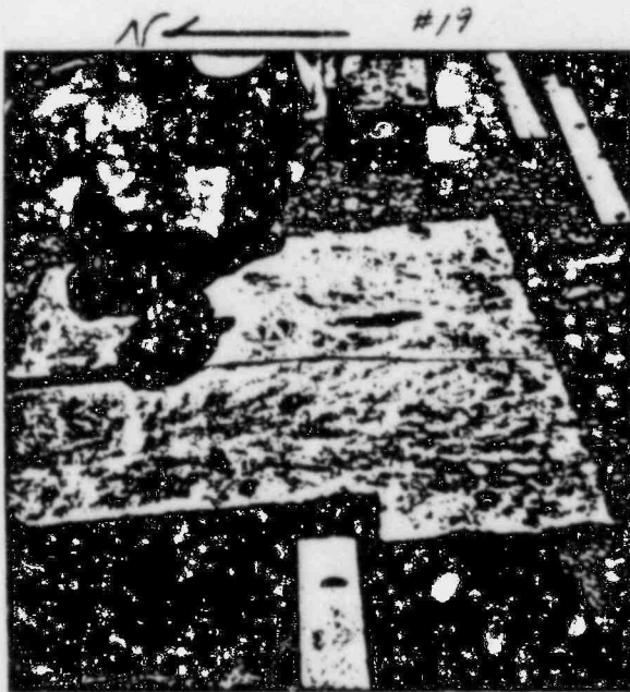
6/29/83 PLATE No. 4 (SOUTH END) NO CONCRETE CUT, 4 NIPPLES FOR RATE, WOOD BULKHEAD
