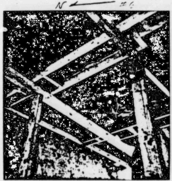
6/28/83 WOODEN BULKHEAD AT RATES #2 & #3. BOTH WITH LEAD WOOL/EXP. METAL BEHIND
