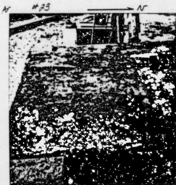
7/2/83 RATE No. 5A (SOUTH END) SECOND DRYPACK TEST RATE AT SAME LOCATION ALSO USING MASTERFLOW #713
