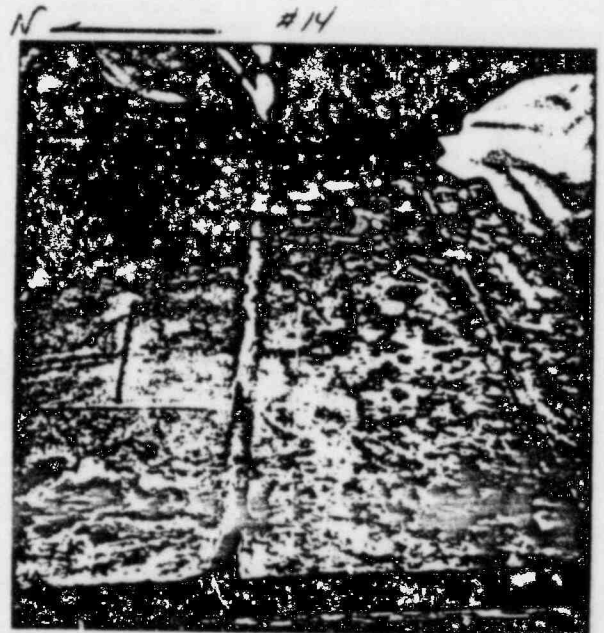
6/29/83 RATE No. 1 (SOUTH END) CONCRETE CUT PARALELL LINES, 4 NIPPLES FOR RATE, WOOD BULKHEAD
