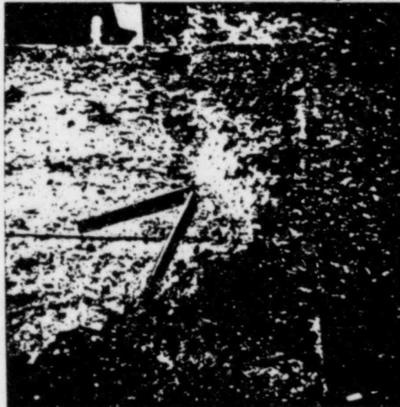
7/7/83 PLATE No. 5B (NORTH WEST CORNER) APPARENT LOSS OF CONTACT AREA 2'11" x 6". THE P.B. APPEAR TO HAVE SLIPPED ON THE WEST SIDE (1 1/2" TO 2" GROUT PAD)
