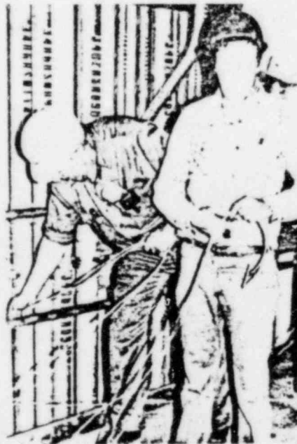
Pulling cable for fire detection and alarm system, electricians Jim Mathew, left, and Dave Frumveller.
