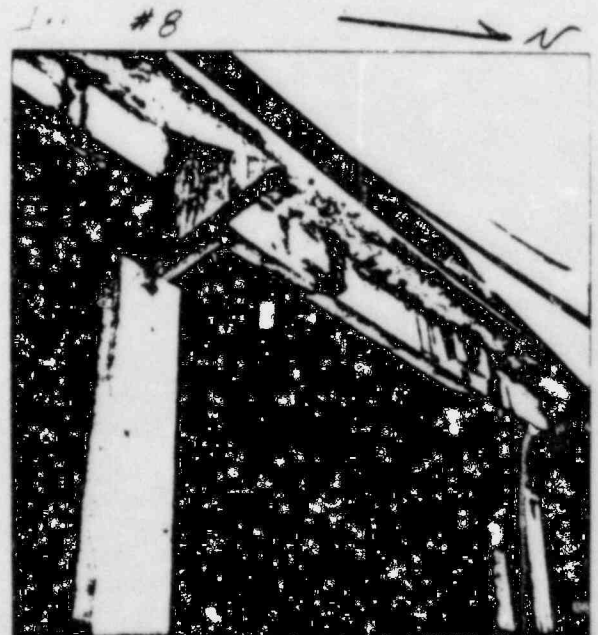
6/28/83 WOOD BULKHEAD WITH AIR VENTS PLUGGED @ EAST SIDE OF RATE No. 4. RATES SUPPORTED BY ANCHOR BOLTS ONLY
