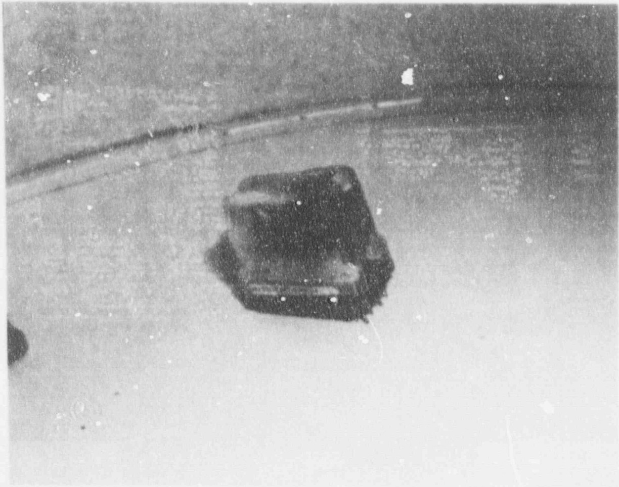
Figure 4-26. Overheated Degraded Condition of Struthers-Dunn 219 Control Relay
