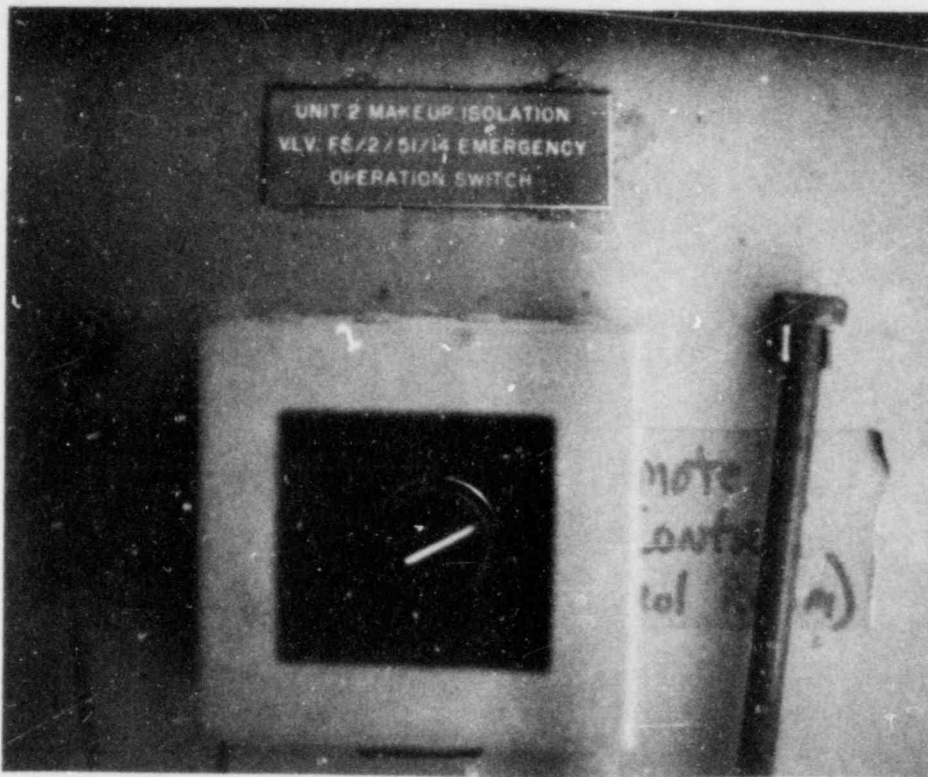
FIGURE 4.6. Actuation Switch for the Makeup Control Valve to the High-Pressure Injection System - cover closed
