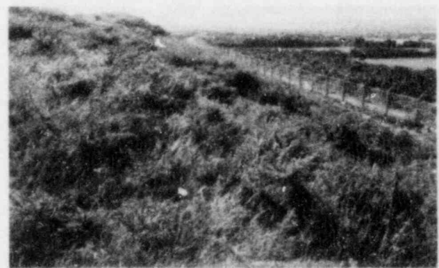
d. A completed Earth Mounded Concrete Bunker at the Centre de la Manche, France. Upon completion of backfilling operations, the entire mound is covered with a thick layer of impermeable clay, which in turn is covered by a layer of topsoil. The surface of the mound is stabilized by planting native vegetation which not only stabilizes the soil but encourages drying.
