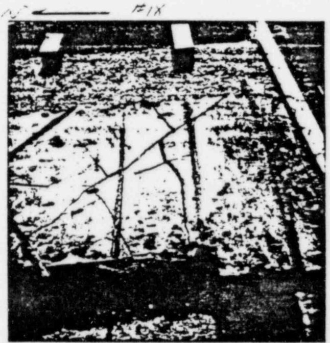
6/29/83 PLATE No. 3 (SOUTH END) CONCRETE PARALELL LINES, 4 NIPPLES FOR RATE, LEADWOOL/EXP. METAL BULKHEAD
