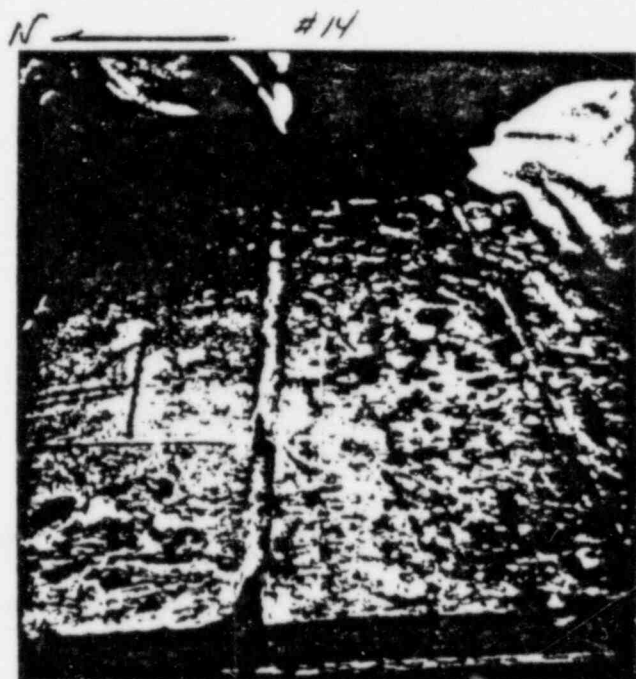
6/29/83 PLATE No. 1 (SOUTH END) CONCRETE CUT PARALLEL LINES, 4 NIPPLES FOR RATE, WOOD BULKHEAD
