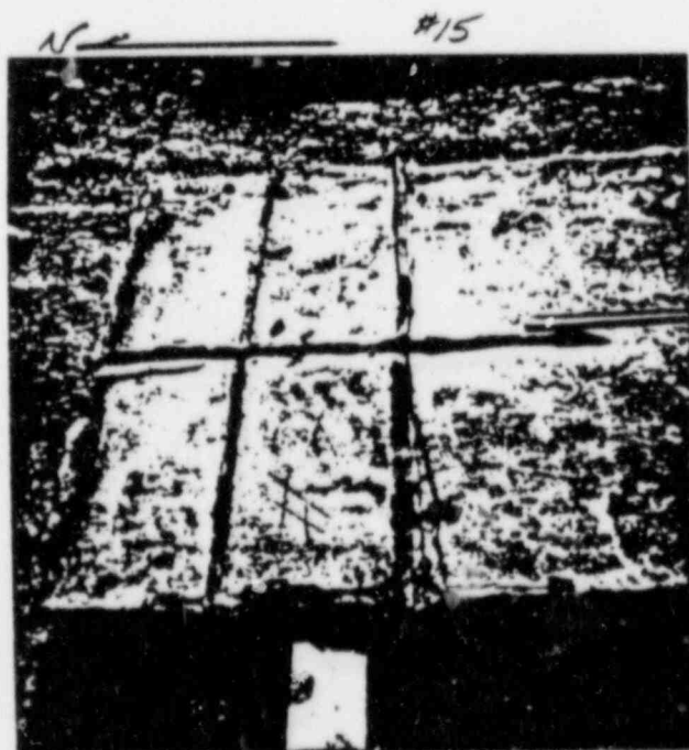
6/29/83 PLATE No. 2 (NORTH END) CONCRETE CUT "H" PATTERN LEAD WOOL/EXP. METAL BULKHEAD 4 GROUT NIPPLES FOR WIND RATE
