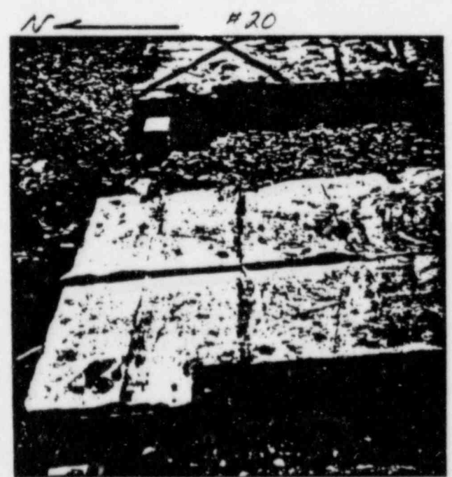
6/29/83 PLATE No. 4 (NORTH END) CONCRETE CUT "H" PATTERN, 4 NIPPLES FOR RATE, WOOD BULKHEAD
