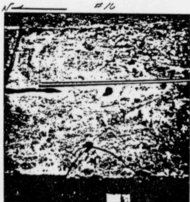
6/29/83 PLATE No. 2 (SOUTH END) NO CONCRETE CUT, 4 NIPPLES, LEAD WOOL/EXP. METAL BULKHEAD
