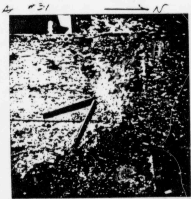
7/7/83 PLATE No. 5B (NORTH WEST CORNER) APPARENT LOSS OF CONTACT AREA 2 1/2" x 6". THE N.B. APPEAR TO HAVE SLIPPED ON THE WEST SIDE. (1 1/2" TO 2" GIRT I.P.)
