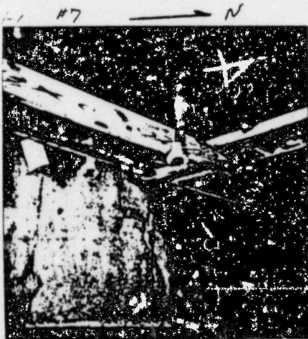
6/28/83 TYPICAL GROUT NIPPLE SET-UP WITH C.P. COUPLING, PIPE NIPPLE, VALVE AND WELDED NIPPLE. (SHOWN @ RATE No. 4)
